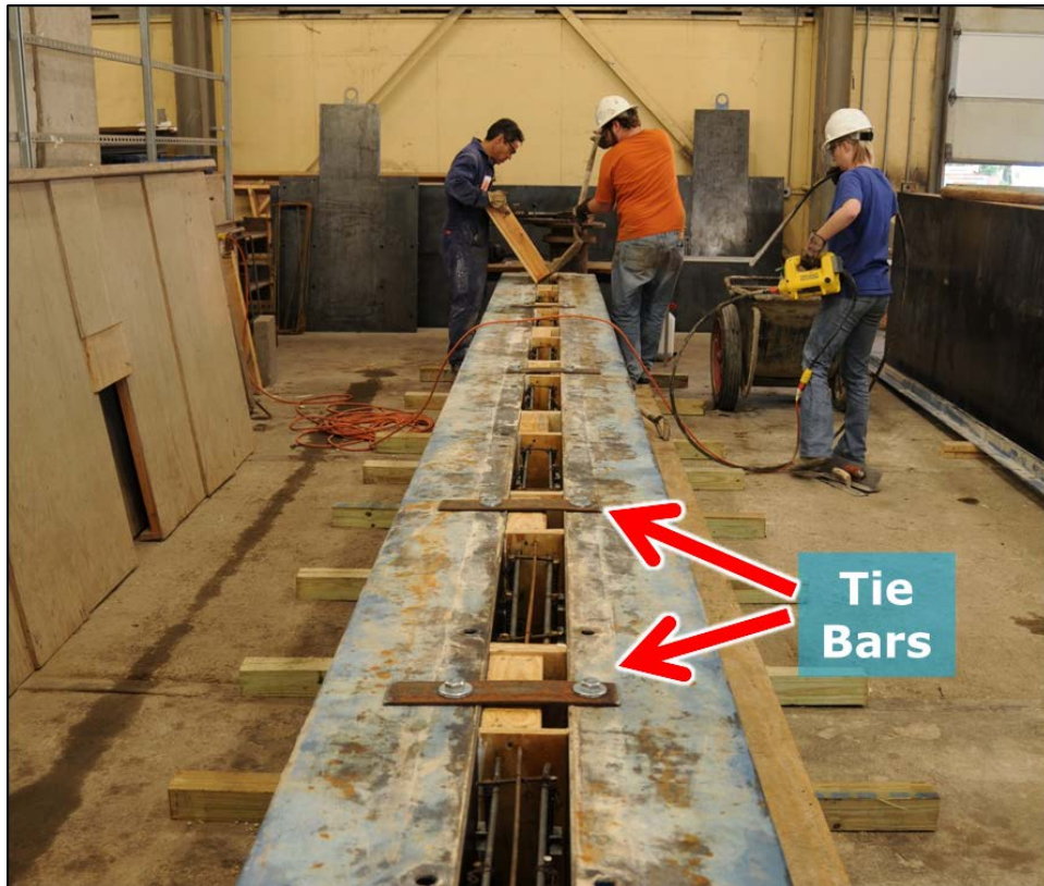
Figure 3-4: Side Form Tie Bars
