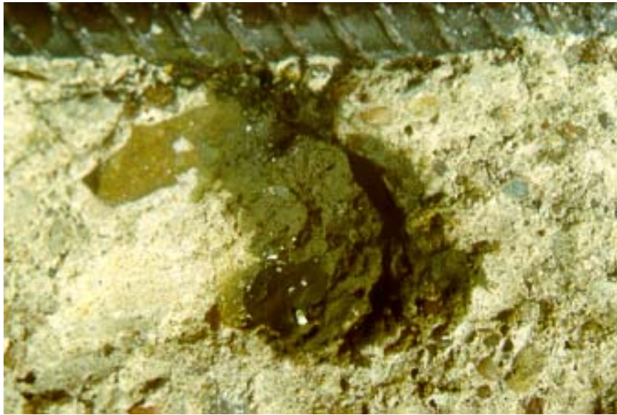
Figure 5.8. Green Corrosion Fluid on Beam 34.
