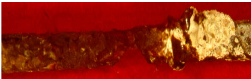
Figure 5.15. Significant Loss of Bar Area (Beam 19).
