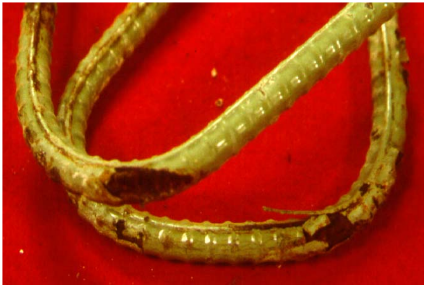
Figure 5.22. Corrosion Damage on Stirrup (Beam 30).
