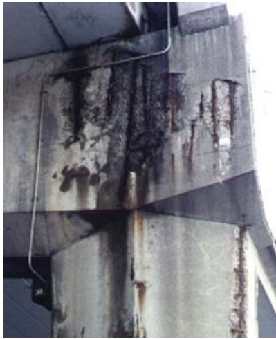
Figure 1-1 Damage to a Reinforced Concrete Structure ( www.corrosion-club.com )
