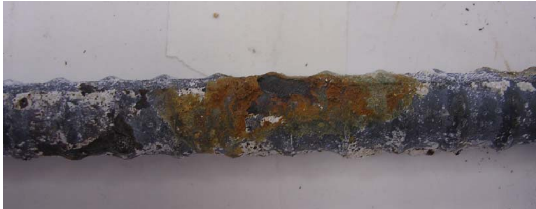
Figure 4-10. Heavy reinforcement degradation caused by corrosion
