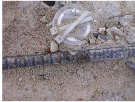
(b) Observed corrosion of reinforcement in vicinity of basic sensor
