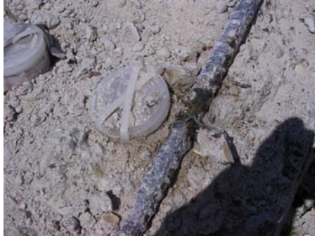
(a) Observed corrosion of reinforcement in the vicinity of improved sensor
