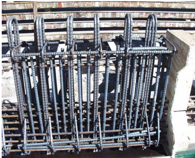
Figure 3.2: Congestion of Reinforcement at End of Beam
