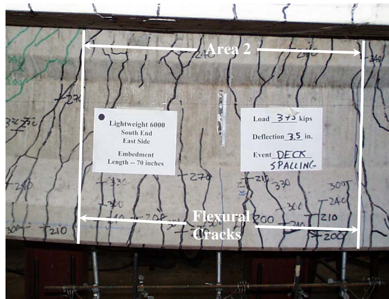
Figure 5.25: Zone 2 – Cracking Pattern
