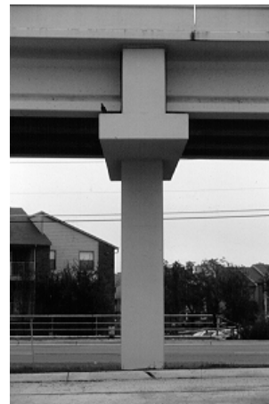
Figure 5.66 Balanced appearance of a column and bent cap stem of equal width
