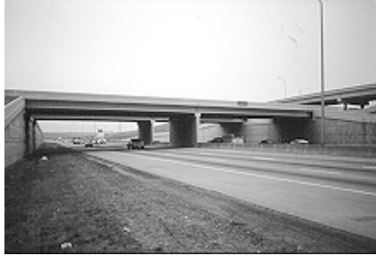
Figure 5.8 A wall substructure unit used for a highway overpass
