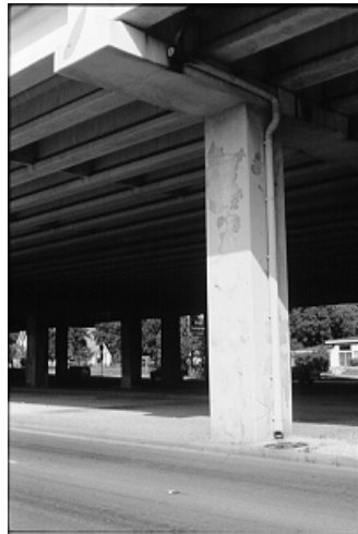
Figure 5.58 Unattractive peeling of painted concrete
