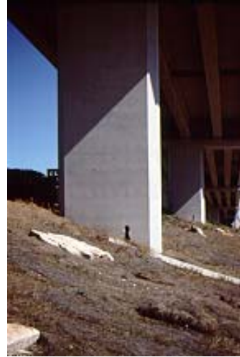
Figure 3.25b Outlet of an internal drainpipe
