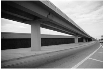
Figure 5.15 A hammerhead bent cap fully integrated into the depth of the superstructure through the use of dapped girders
