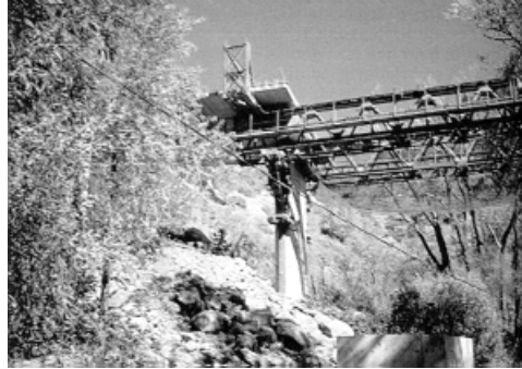
Precast segmental superstructure placed on erection trusses using a launching gantry from the already built deck
