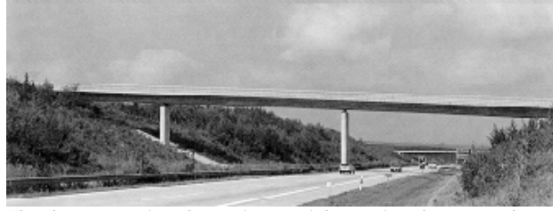
The clear expression of a continuous girder on pinned supports shows the lack of moment transfer between the super- and substructure
