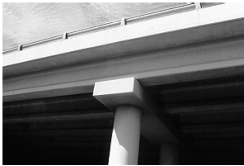
Figure 5.65 Inverted T bent cap stem shaped to mimic the concrete I-girders it supports
