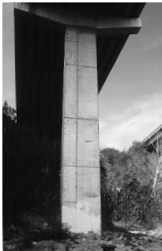
Figure 1.8 Lack of attention to concrete finish results in an unattractive pier.
