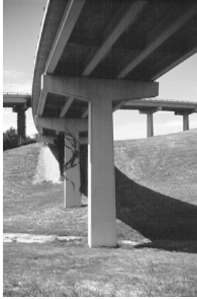
The tapered cap and column of this hammerhead bent is structurally expressive of the increased moment resistance required at the cap/column intersection and at the column base under critical loads
