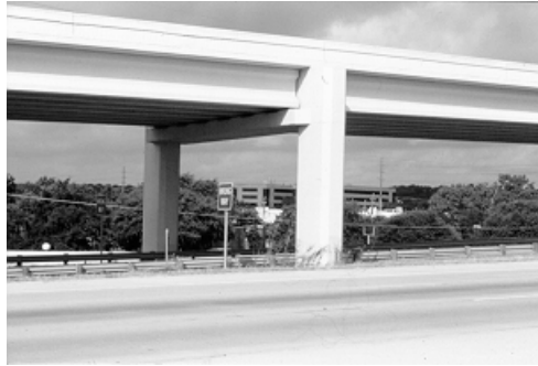
Figure 5.63 Continuation of chamfers from column to bent cap for a well-integrated form.
