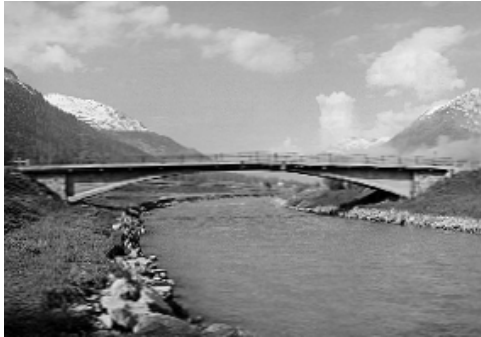
Cracks appeared in the side walls of this three-hinged box-arch when the bridge was put in service.
