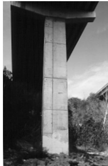
Figure 3.63 Lack of attention to concrete finish detracts greatly from the overall bridge form. These piers are heavily viewed from a popular hike & bike trail
