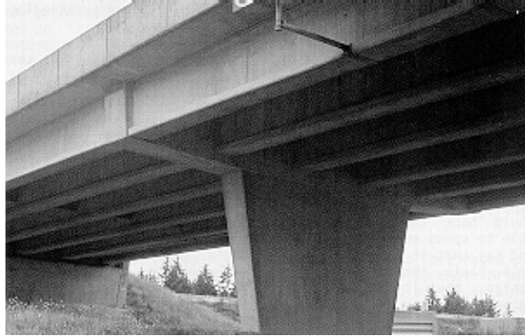
Figure 5.40 A fully integrated cap provides a clean transition between the superstructure and substructure
