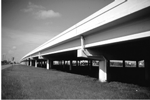
Figure 3.25a Drainpipes tacked onto the substructure
