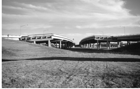
Figure 6.21 Stubs-outs on the south end of the US 287 project (view looking south)
