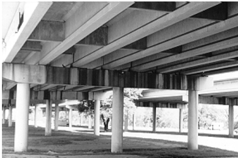
Figure 3.26 Substructure staining due to the open joint above
