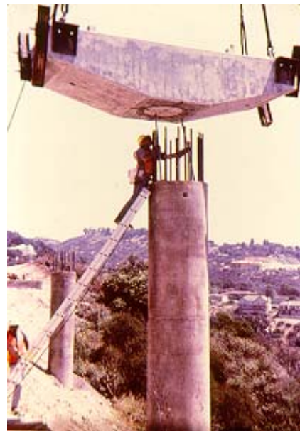
Figure 4.9 Placement of a precast pier cap on a cast in place column
