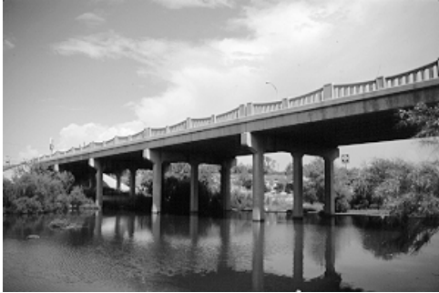
Figure 6.4 One of the older bridges crossing the Concho River in San Angelo
