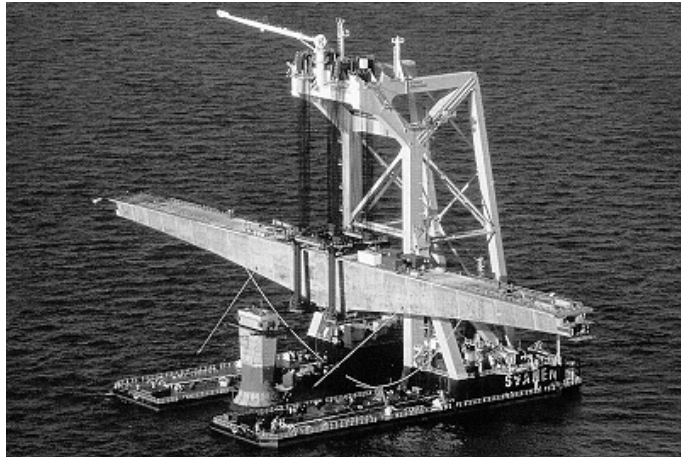
Figure 4.20 Placement of a 200m (655') precast segmental girder for the Northumberland Strait crossing. 40
