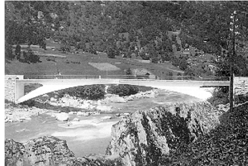
The side wall material not required structurally was removed from this three-hinged arch resulting in a new, elegant, and more efficient form.
