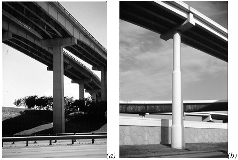
Figure 5.30 A subtle column taper (a) is more attractive than abrupt changes in cross section (b) for tall columns
