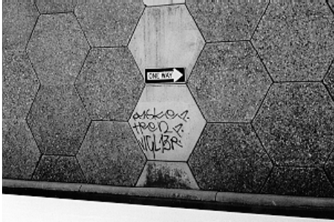
Figure 5.46 Exposed aggregate finishes may be less likely to attract graffiti than plain concrete.
