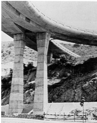
These tall piers are more fixed at the base than at the top. Under critical lateral loads, the point of inflection is located at about two-thirds the height from the base, allowing the columns to taper in at that location of minimum moment. 78
