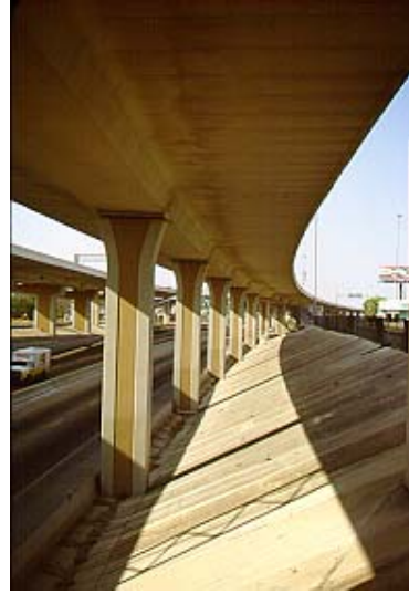
Figure 4.4 The San Antonio "Y" project in Texas shows off the elegance possible with segmental concrete bridge design
