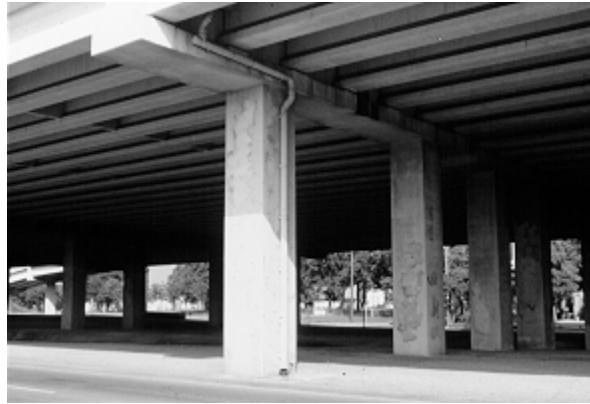
Figure 3.21b Tacked on drainpipes and peeling paint create a feeling of decay
