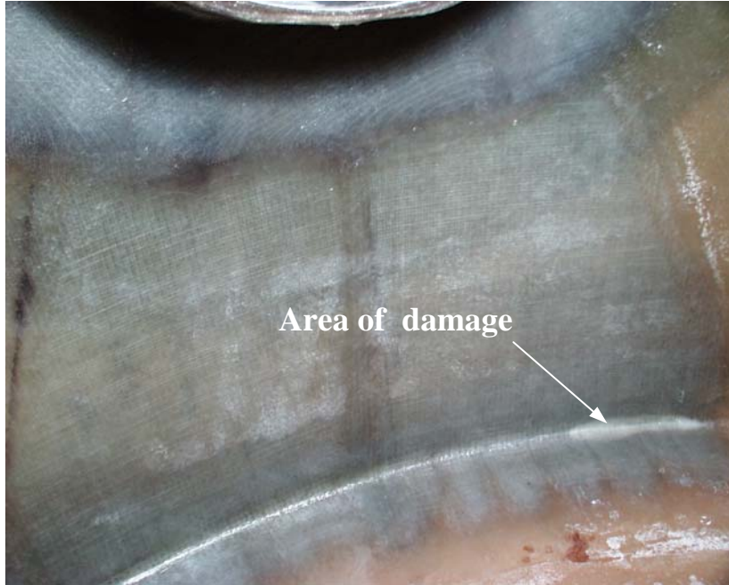
Figure 10.47 – Damage to interior reinforcement at intersection of vessel wall and vessel base
