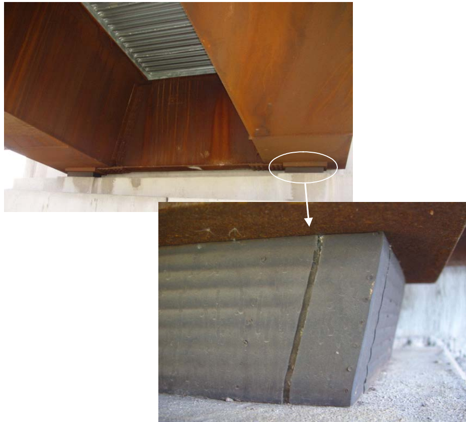
Figure 6.18 Lateral displacement of an end support of the “U.S 290-Bridge”
