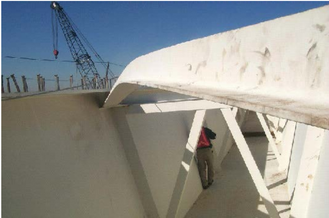
Figure 1.4 Failure of bracing member during construction (Chen, 2002)
