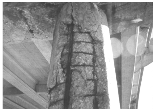
(b) Column Corrosion
