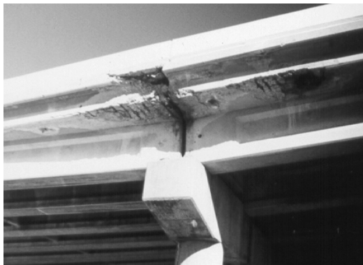
(a) Corrosion at Leaking Deck Joint
