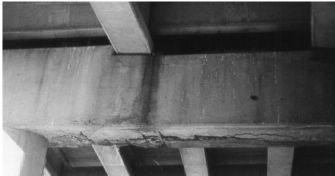
(c) Bent Cap Corrosion
