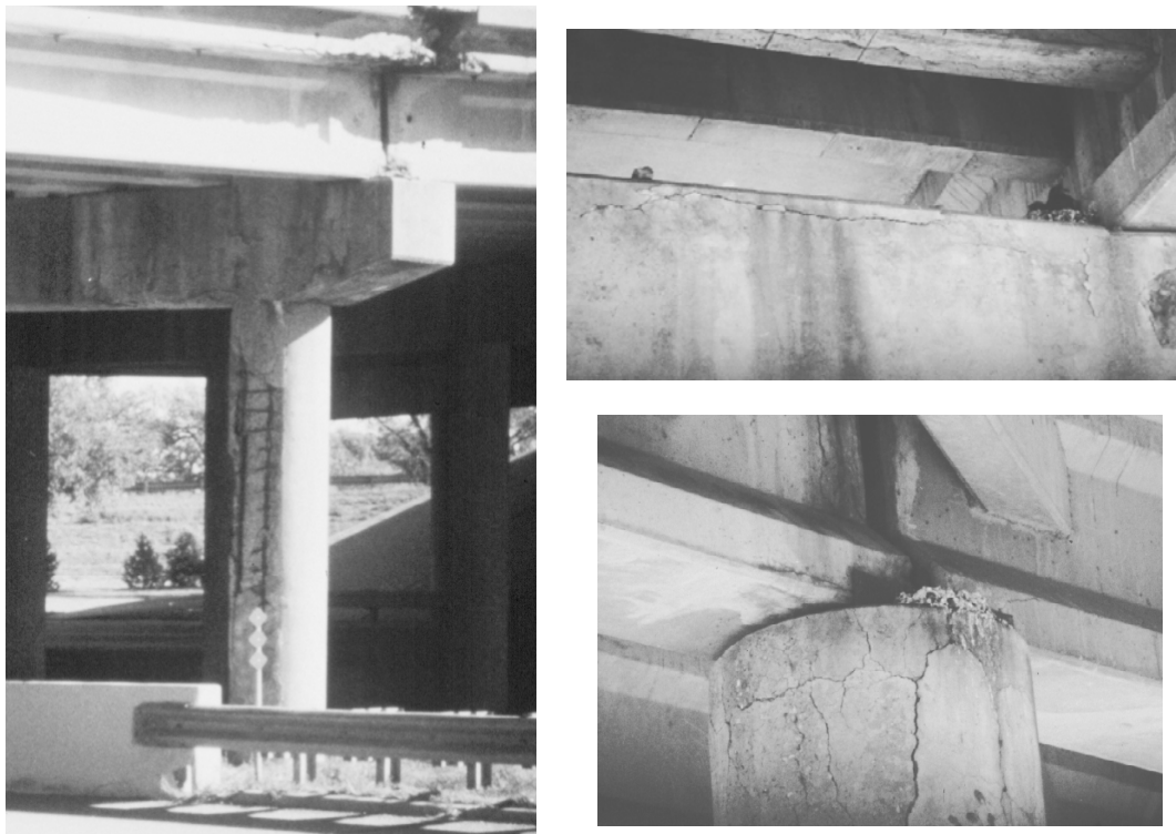
Figure 2.23 - Severe Substructure Corrosion Damage Due to Defective Expansion Joint
