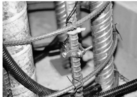
Ground Clamp to Attach Ground Wire
