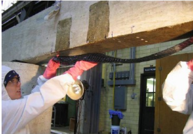
Figure 2-1 Installing a CFRP strip on the tensile substrate of a concrete member
