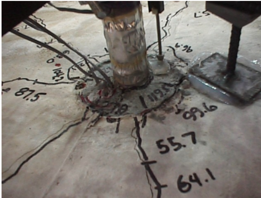
Figure 7.2: GVD03 Cracking at Top of Grout
