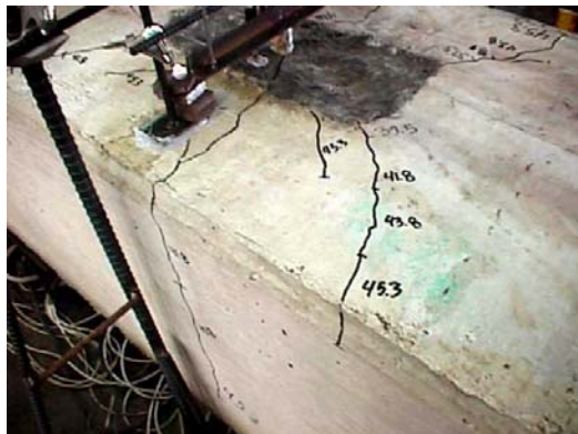
Figure 5.2: Pocket Corner Cracks
