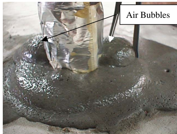
Figure 4.20: Air Bubbles at Grout Surface
