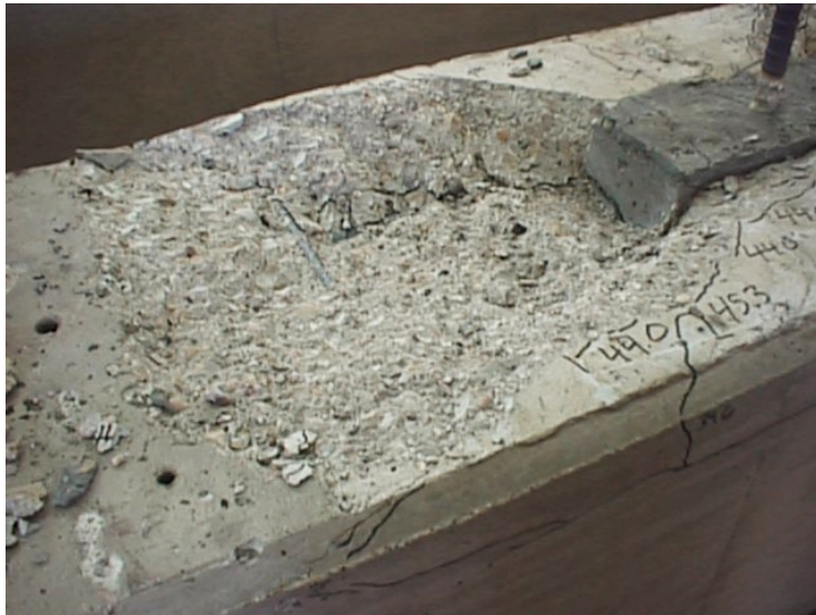
Figure 5.4: Surface Cone Spalling
