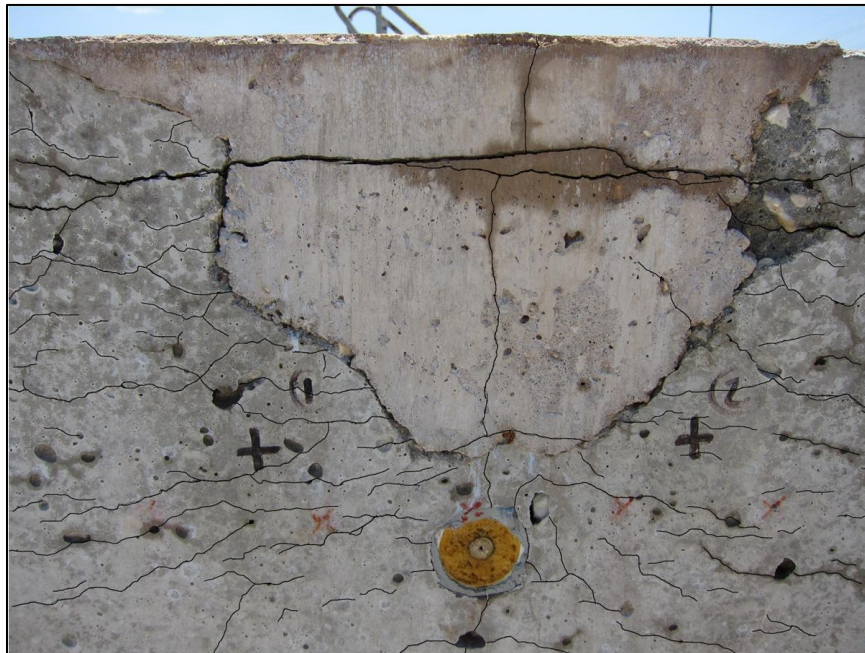
Figure 4-9: Surface Cracking at Location of Fractured Stirrup
