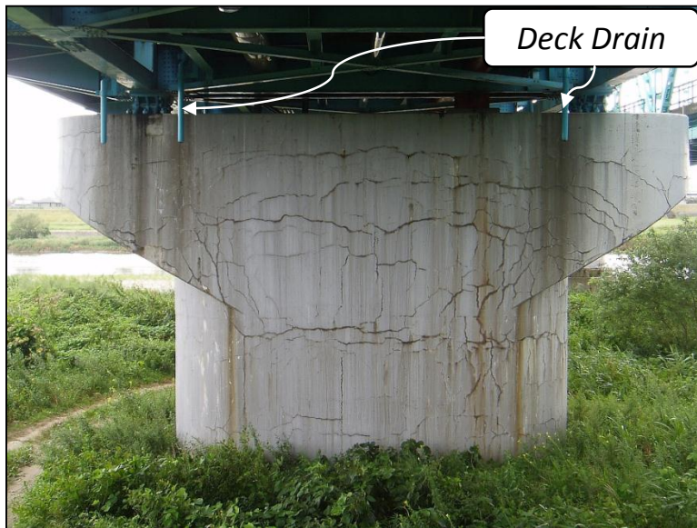
Figure 2-7: Heavily Damaged Bridge Pier with Confirmed Reinforcing Bar Fractures (Daidai and Torii 2008)
