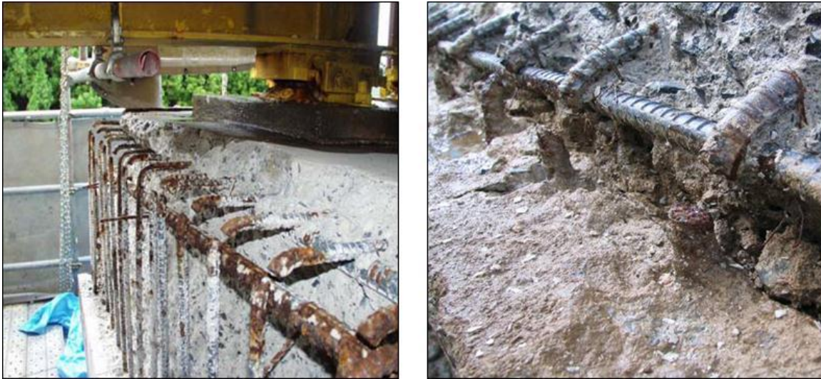
Figure 1-1: Examples of ASR-Induced Reinforcing Bar Fracture in Japan (Torii et al. 2008)
