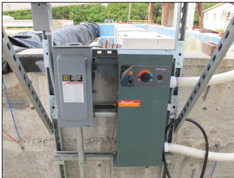
Figure 3-10: Electric Water Heater for High Temperature Conditioning
