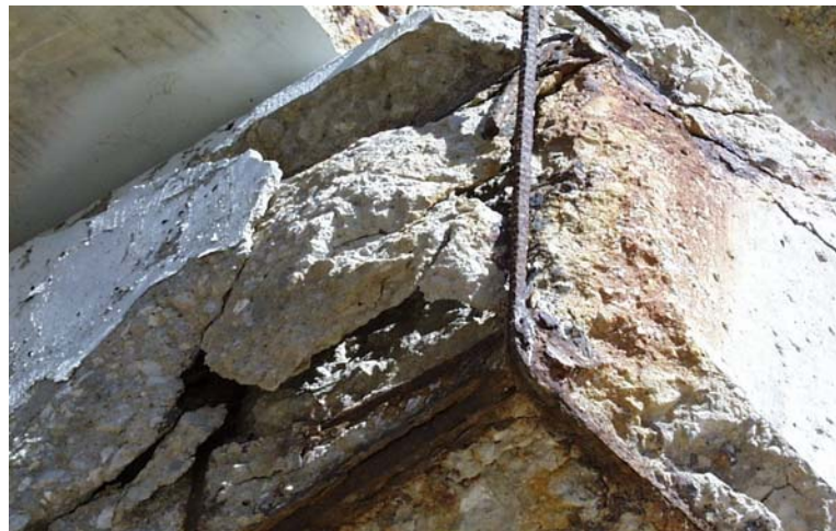
Figure 4.2 Closeup of corrosion damage on Structure #8.
