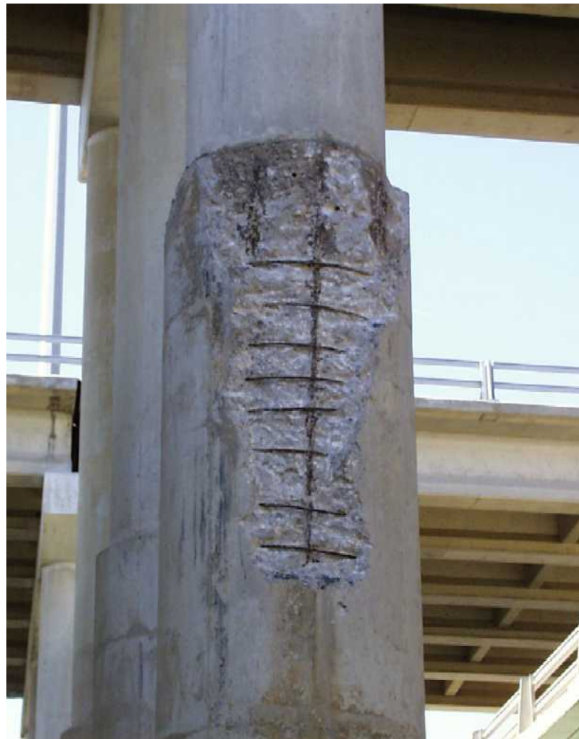
Figure 5.3 Concrete spalling on a bridge support column.
