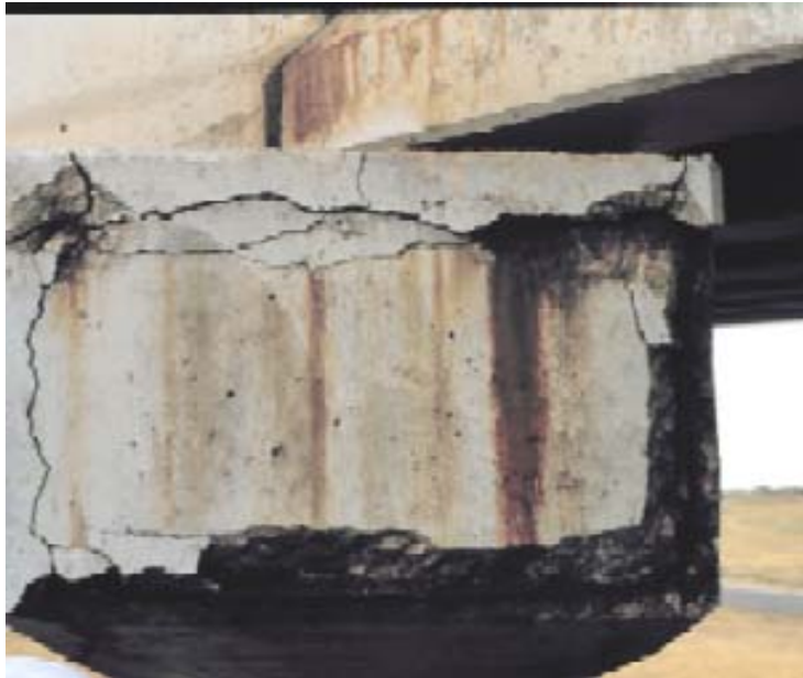
Figure 5.1 Corrosion damage on downstream endcap.
