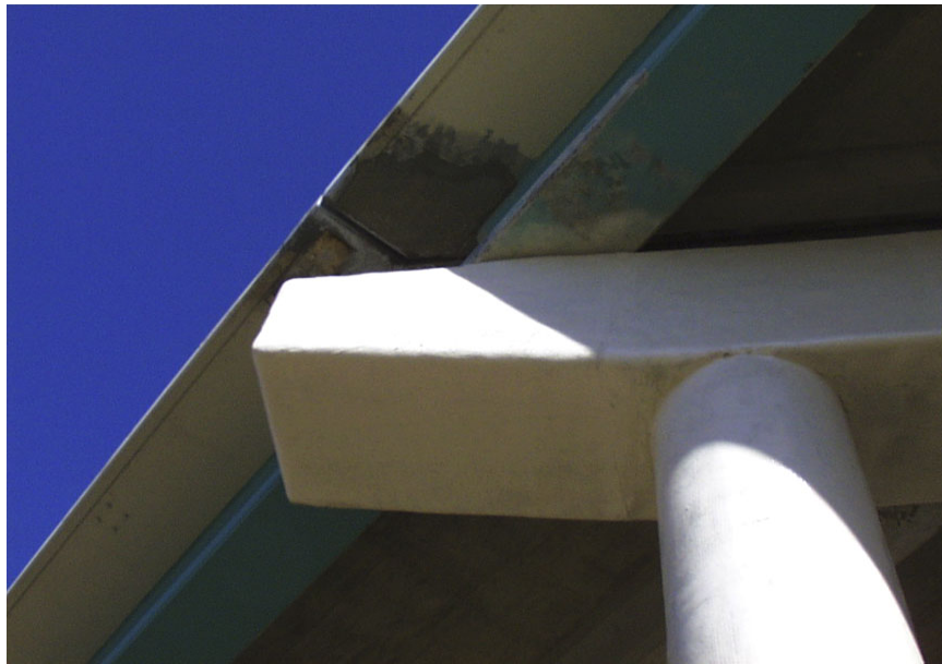
Figure 4.9 Wrapped and painted endcap on Structure #2.
