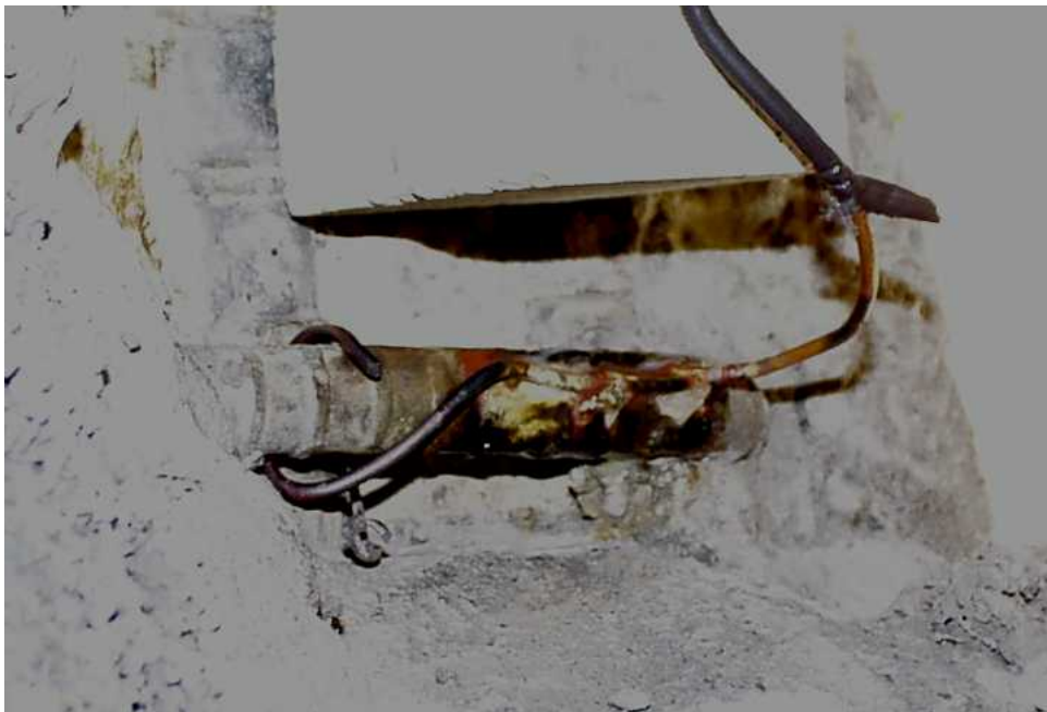
Figure 5.11 Typical silver soldered electrical connection.
