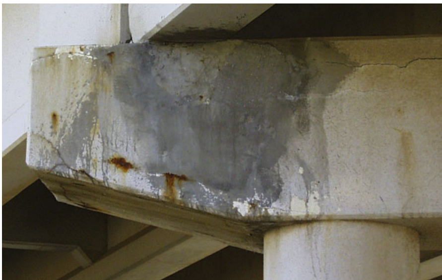
Figure 5.6 Delaminations and corrosion stains on a downstream endcap.
