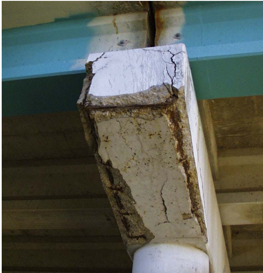
Figure 1.2 Typical Corrosion Damage on Project CSR 783-2-66.
