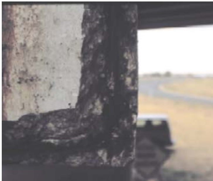
Figure 5.2 Closeup of area with severe concrete spalling.
