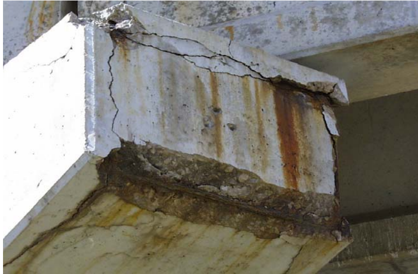
Figure 4.1 Endcap damage to Structure #5.
