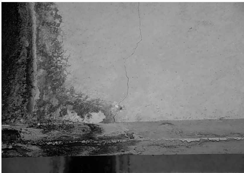
Figure 3.3 Vertical Crack in Girder
