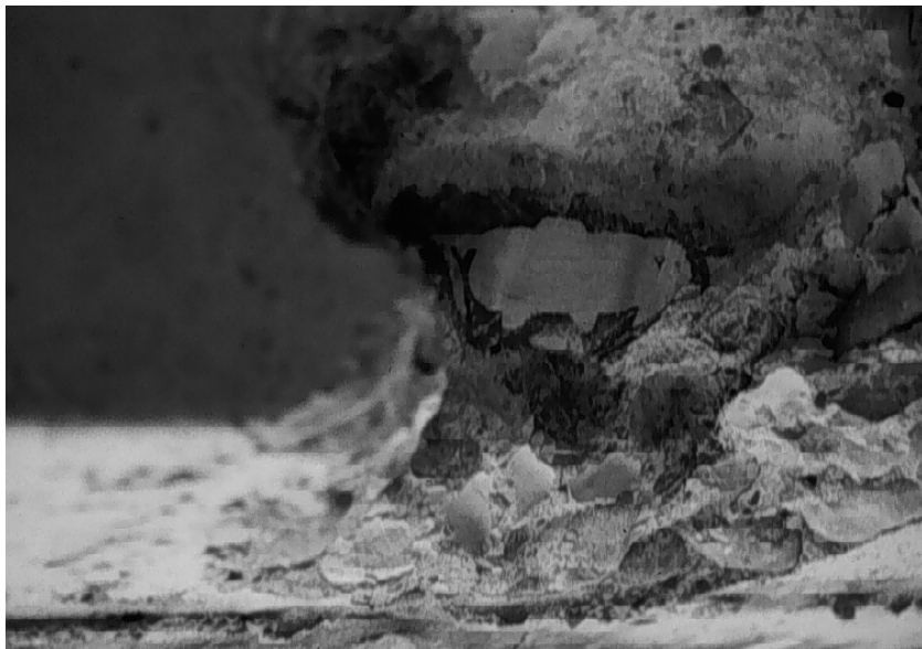
Figure 3.11 Exposed Reinforcing Bar at Mid-span
