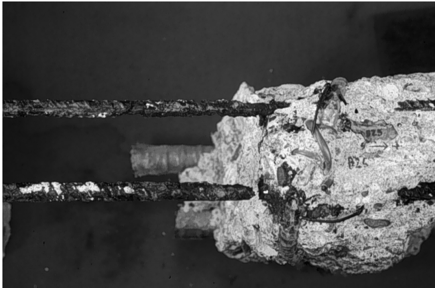
Fig. 9.66: Upper black bar in beam B25 fractured during autopsy at severely pitted location.
