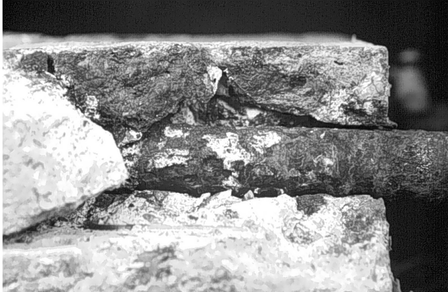
(b) Pitting at straight leg of #8 uncoated bar.
