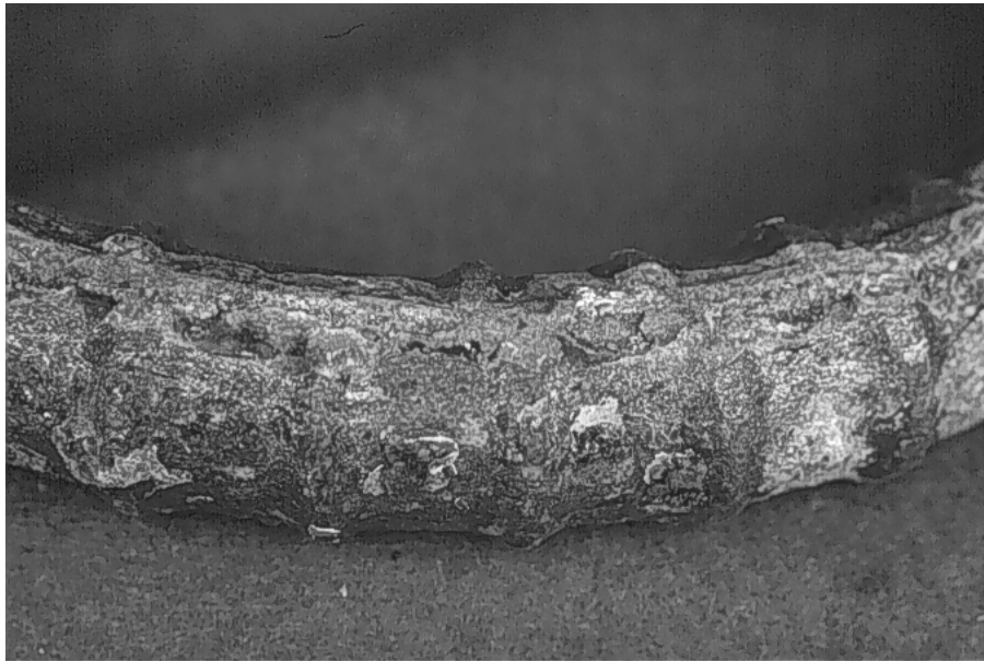
Fig. 8.34: Shallow pitting and accumulation of rust products on steel surface under the coating (outside bend).
