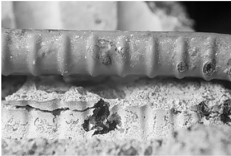
Fig. 8.61: Blisters always formed adjacent to concrete voids.
