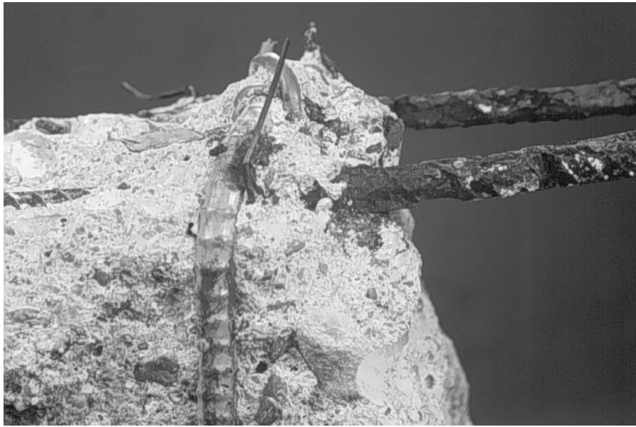
Fig. 9.87: Pitting corrosion of uncoated bars at crack location (beam B25).
