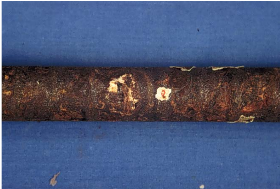
Fig. 9.71: Dark corroded surface on longitudinal upper bar of beam B8 within the wetted region (zone at midspan).
