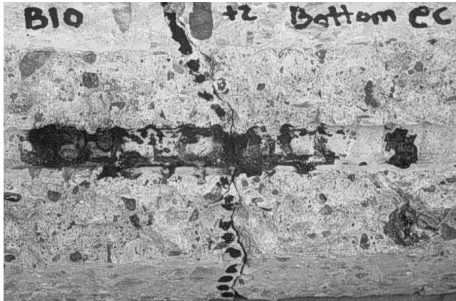
Fig. 9.83: Rust staining on coated bar trace in concrete around crack location at edge of wetted region (beam B10).
