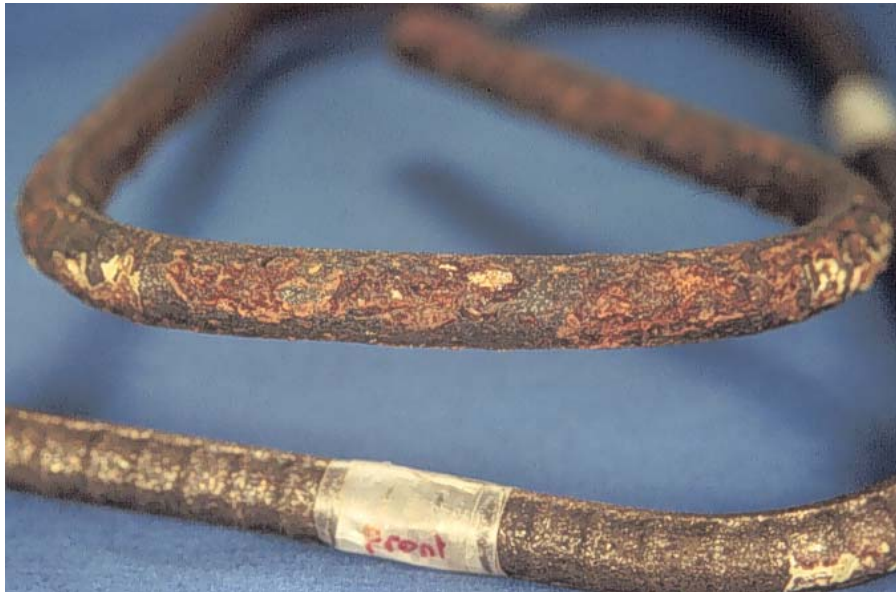
Fig. 9.90: Stirrup leg near the beam front surface (top in photo) is corroded while stirrup hook is mottled (bottom in photo) (Beam B32).
