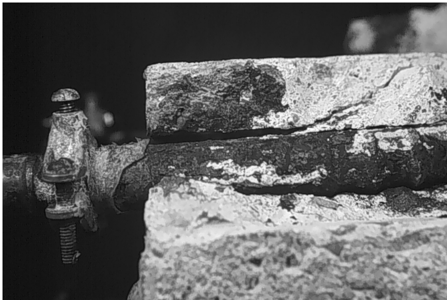
(b) Another aspect of rust inside crack surface.
