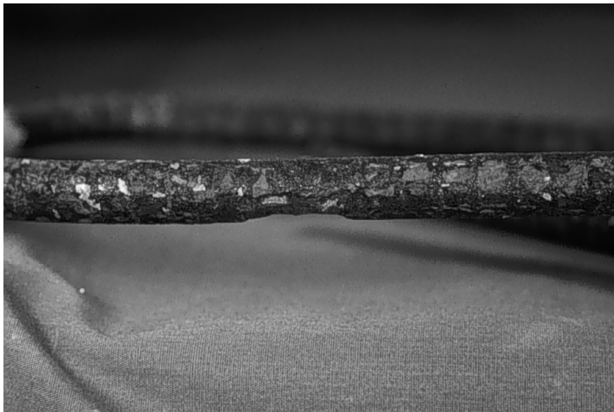
Fig. 9.72: Pitting on stirrup leg near the bottom beam surface (beam B17).
