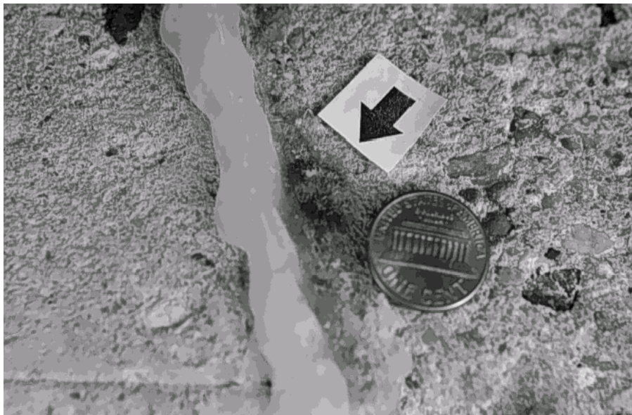
Figure 9.44: Rust spot just outside wetted region on beam B12.
