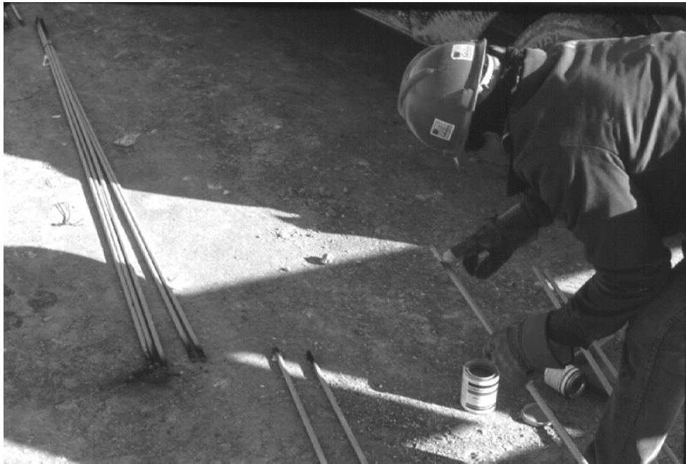
Figure 6.1: Improper field practice: Epoxy coated bars were flame cut and, immediately thereafter, bar ends are being touched up by hand.
