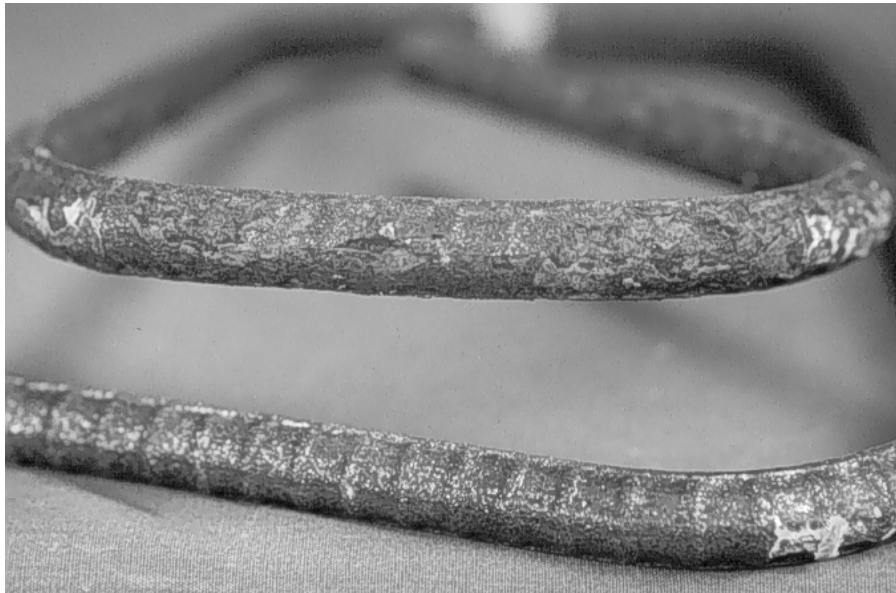
Fig. 9.77: Corrosion on stirrup leg (top in photo) and mottled surface on stirrup hook (bottom in photo). Portion near the front beam surface (beam B32).
