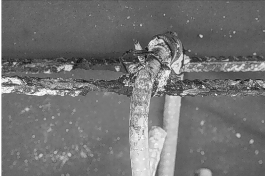
(a) Severe pitting on lower black bar near coated stirrup (beam B23).
