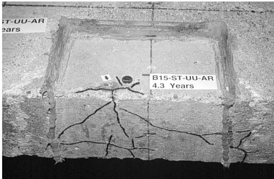
Figure 9.46: Random cracking on front surface of beam B15.
