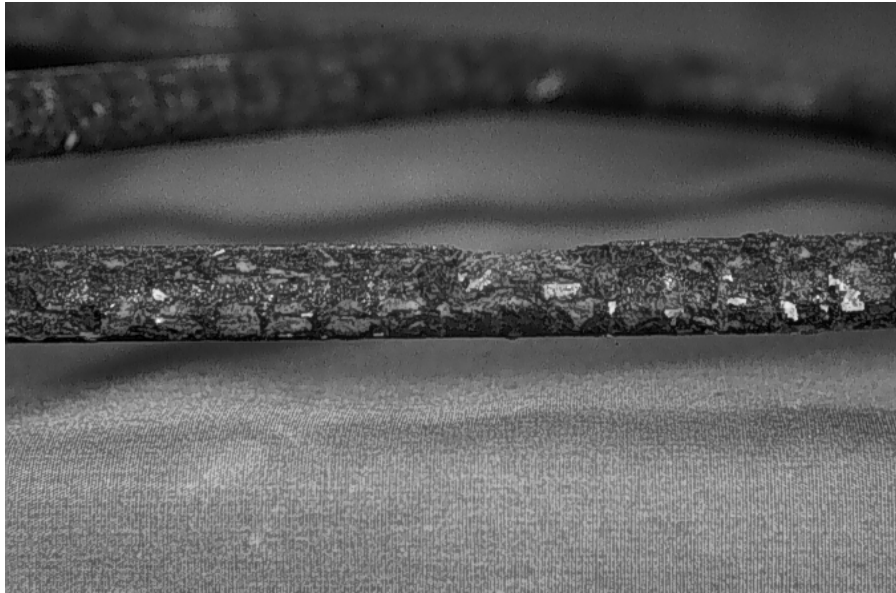
Fig. 9.75: Pitting on stirrup leg near the bottom beam surface (beam B17).
