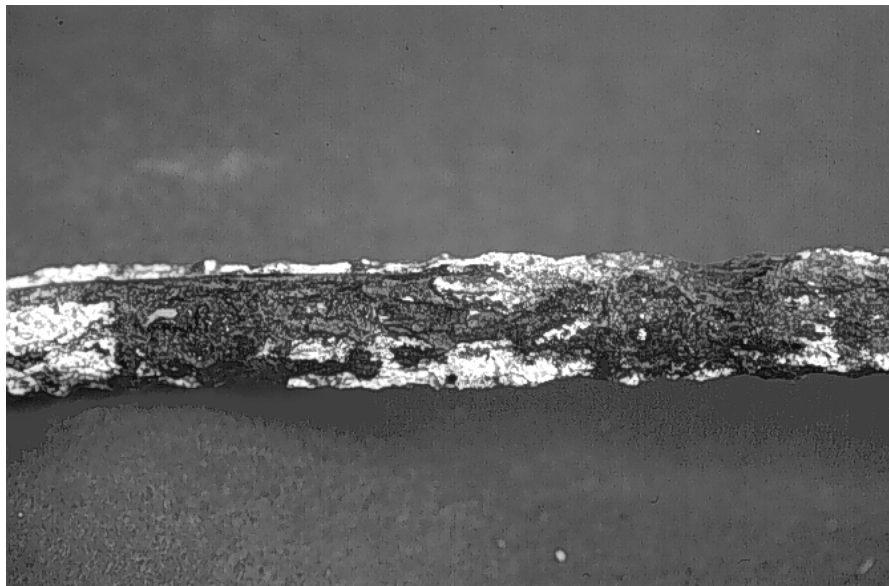
(a) Severe metal loss and pitting at straight leg of #4 uncoated bar.
