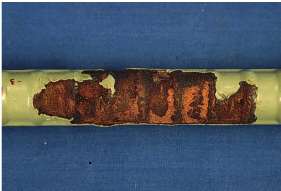
Fig. 9.73: Reddish-brown rust products on lower bar of beam B8 (Zone just outside of wetted region).
