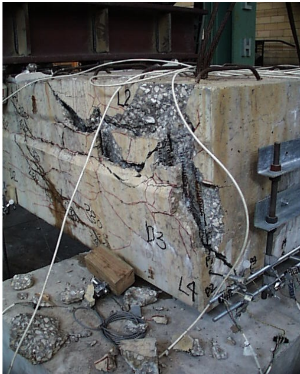
Figure 4.32 - Bearing Failure of BG4S
