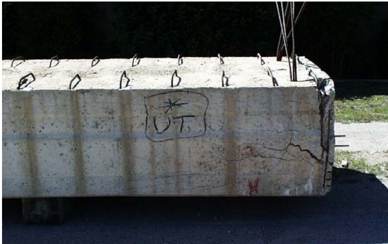
Figure 3.5 - Spalled Concrete on Specimen BG2
