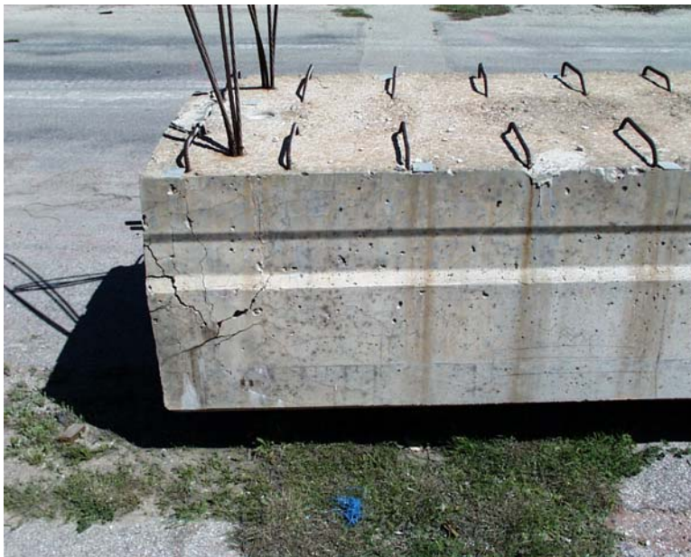
Figure 3.6 - End Damage on Specimen BG2
