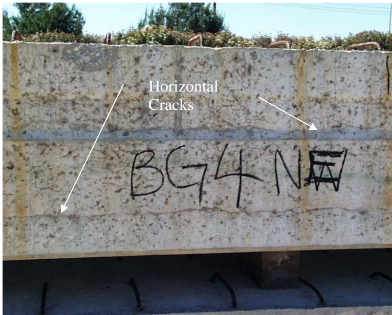
Figure 3.11 - Typical Damage Along the Length of BG4
