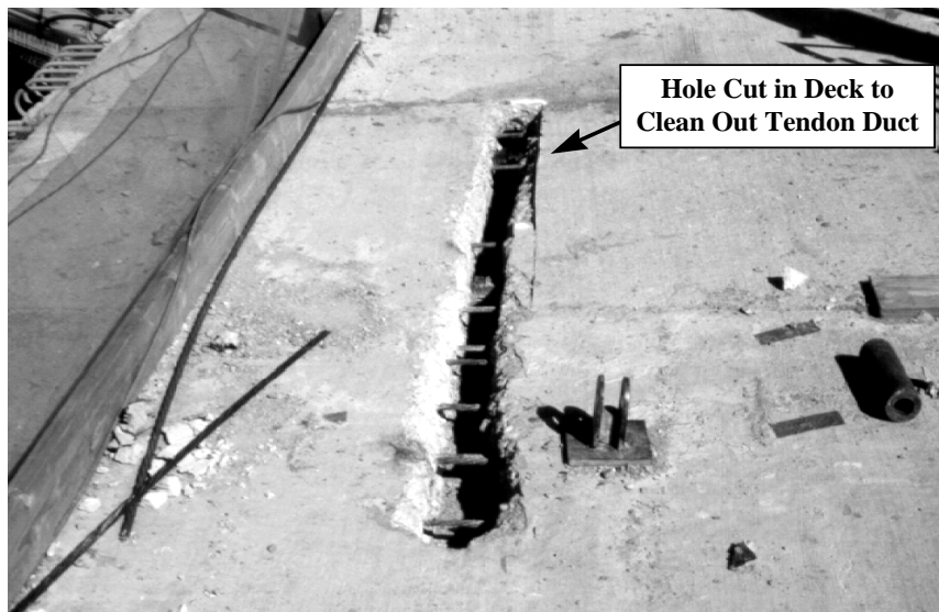
Figure 4.39 - Damage done to the top deck because the cantilever tendon duct became obstructed
