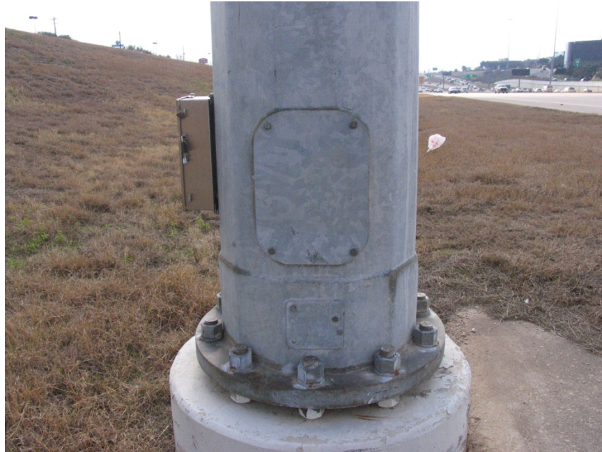
Figure 1.3 Winch System Access Hatch (photo courtesy of Craig Rios)
