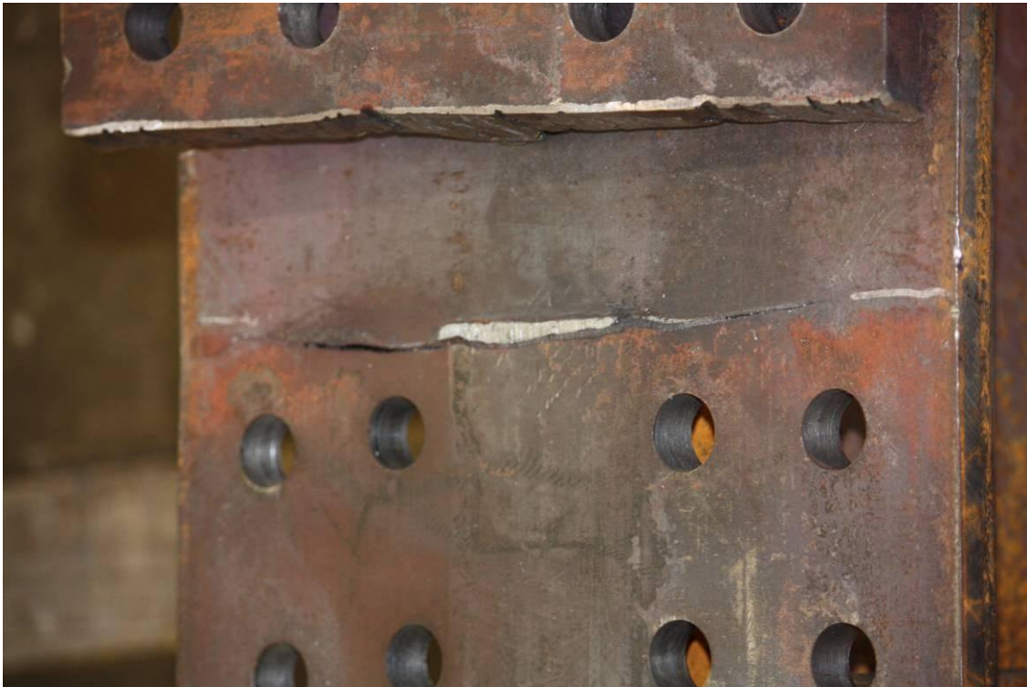
Figure 3-11: Crack on 60A at the edge of the repair plate
