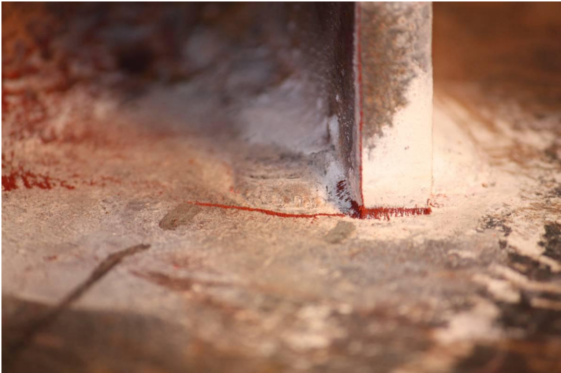
Figure 3-16: Fatigue crack at a perpendicular stiffener on beam 60B
