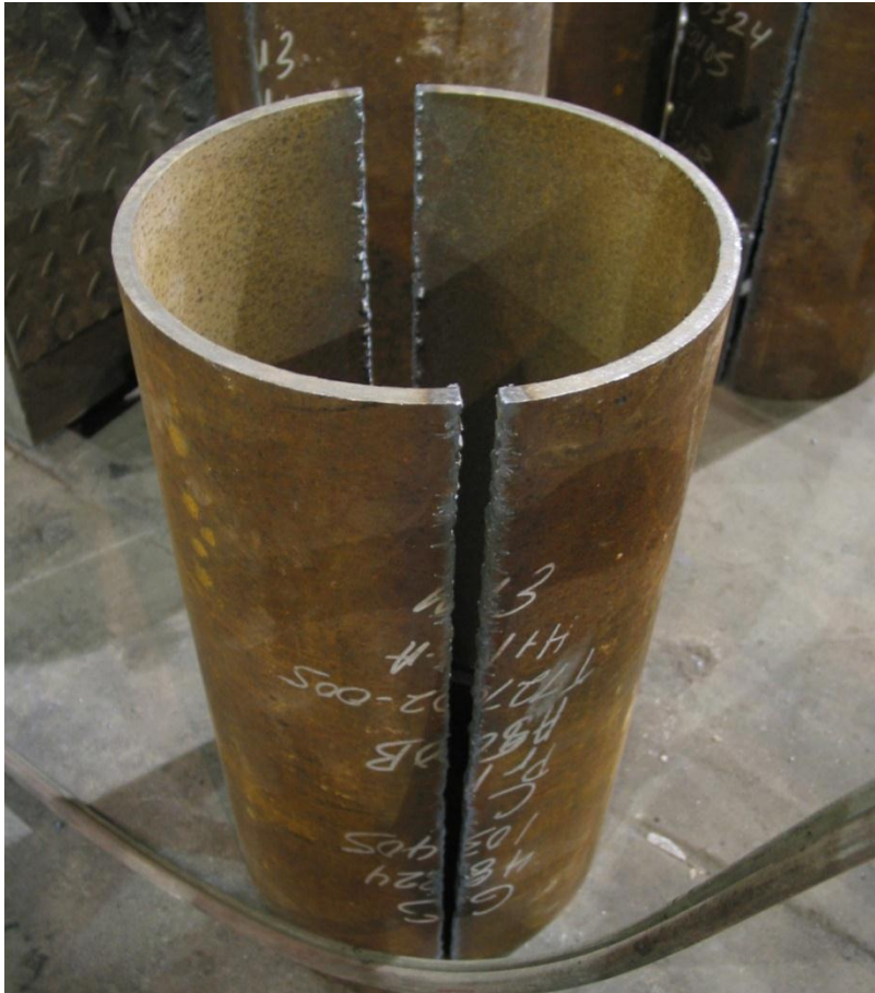
Figure 2-2: A Steel Pipe is Split in Half before Installation on the Girder
