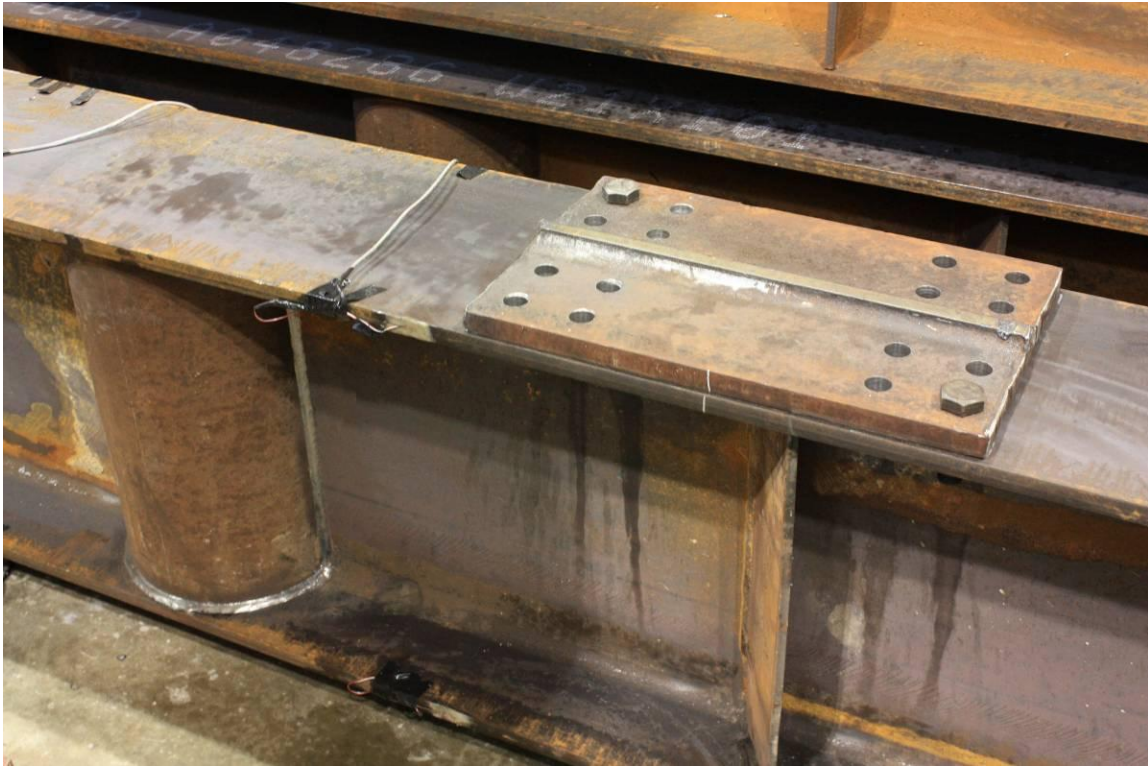
Figure 3-8: A plate is put over the crack surface to prevent the crack from spreading
