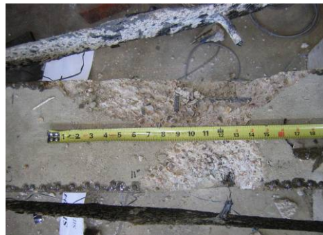
Figure 4.29 Failure mode of Specimen No.4
