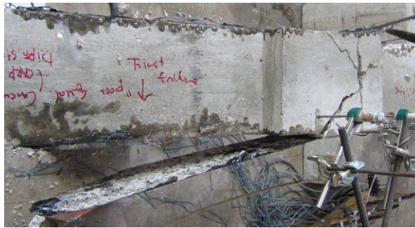
Figure 4.20 Failure Mode of Specimen No.3
