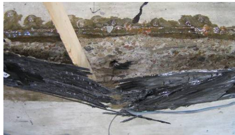
Figure 4.60 Failure Mode of Specimen No.7, Side-A, Fracture of CFRP Anchor
