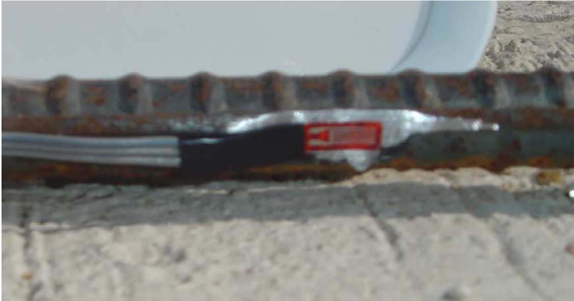
Figure 3-20 Installed Strain Gage on Top Bracing Bar
