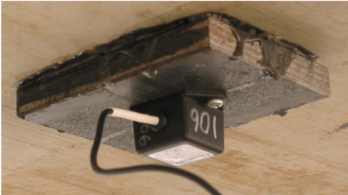
Figure 3-10 Tilt Sensor Attached to Steel Plate
