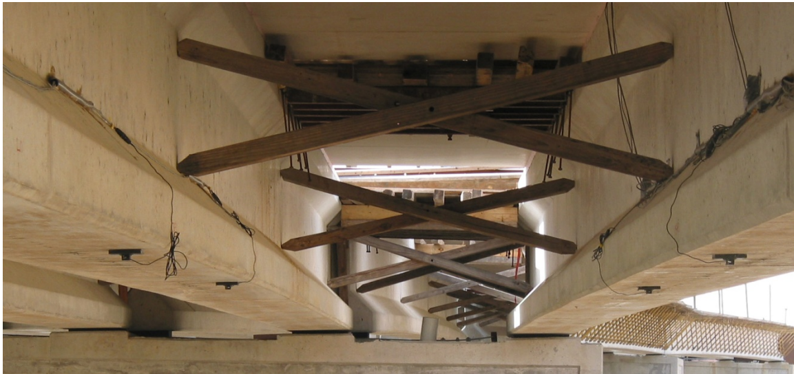
Figure 3-12 Timber Blocking of Concrete Girders
