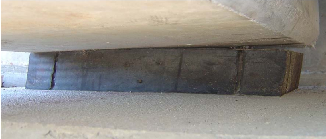
Figure 2-10 Girder Rotates off Bearing Pad
