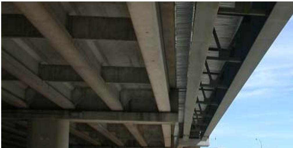
Figure 2-7 Twin Girder Widening with Excessive Girder Twist
