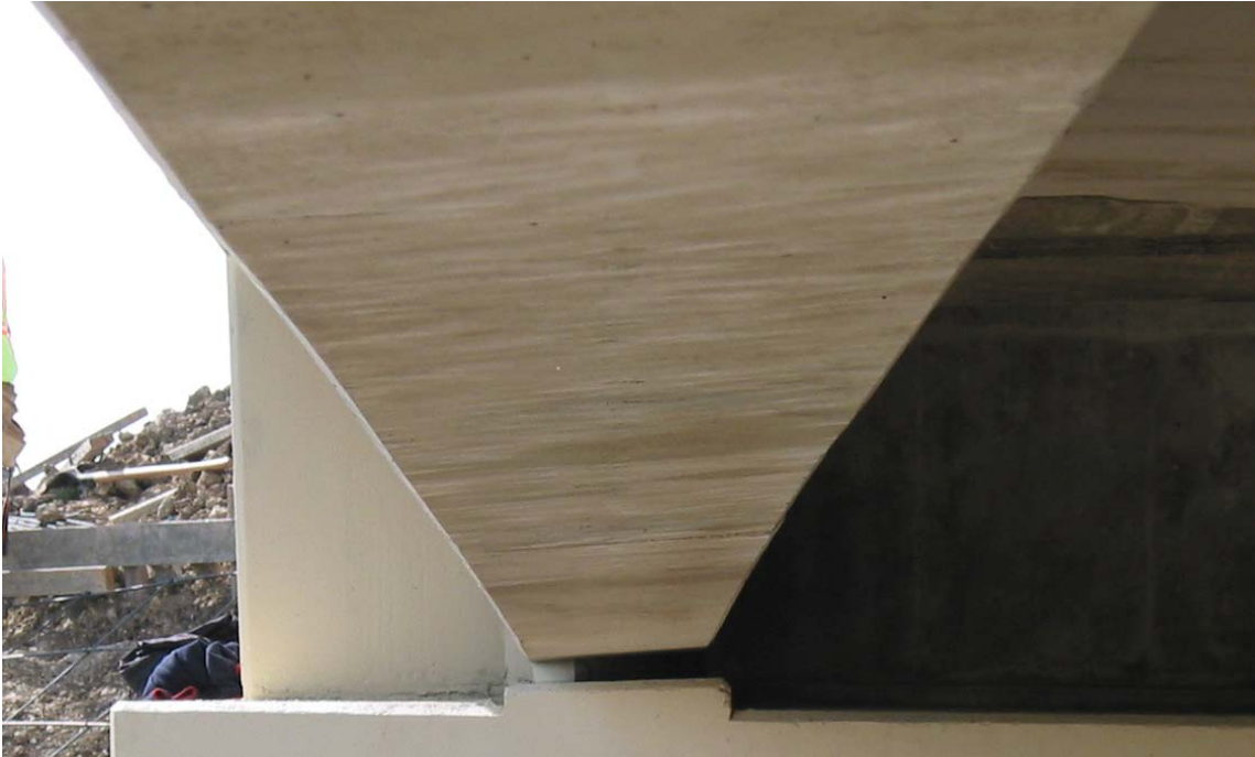
Figure 2-11 Large Rotations of Prestressed, Fascia Girder at Bridge 1
