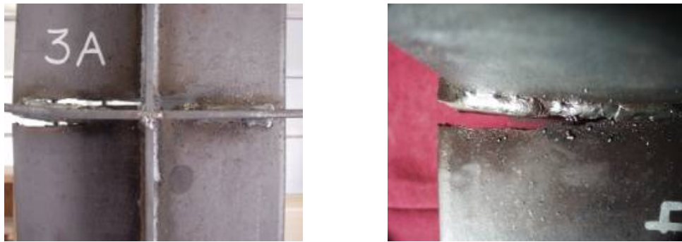
Figure 4-14: Multiple Cracks at Toe of Welds 4T and 4B
