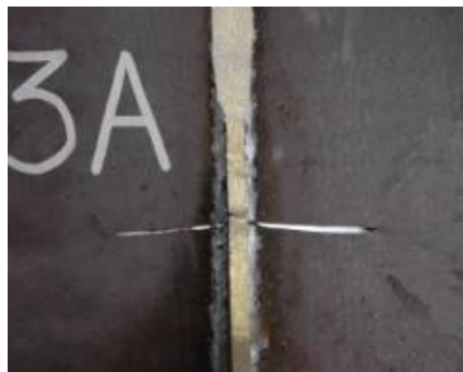
Figure 4-15: Crack at Upper Radial Web Taper
