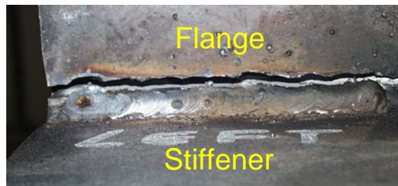
Figure 4-25: Specimen 8C Weld 2T Toe Crack
