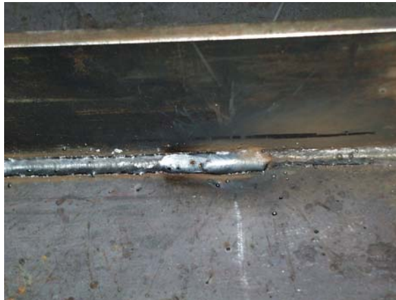
Figure 2-15: Weld Start-Stop Repair
