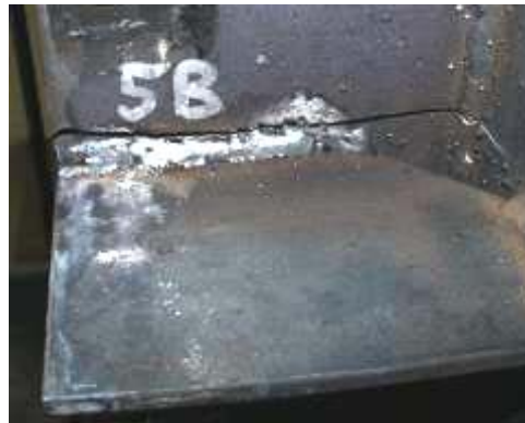
Figure 4-16: Crack at Toe of Weld 2T
