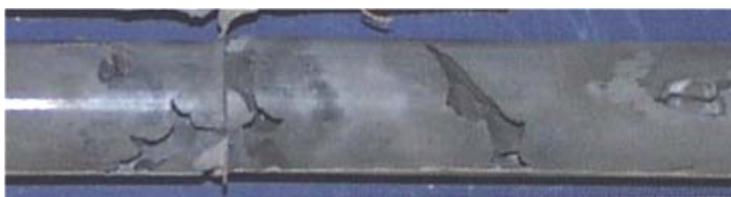
Voids Caused by Lack of Grout Fluidity
