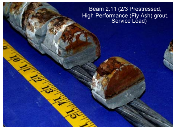
Figure 4.145 Effect of Grout Cracking
