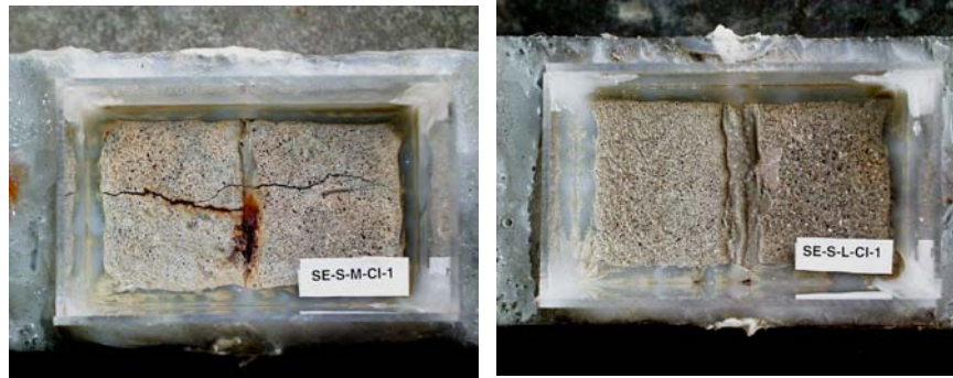
Figure 3.70 Top View of the Effect of a Faulty Epoxy Joint (SE-S-M-CI-1) Compared to a Sound Epoxy Joint (SE-S-L-CI-1)
