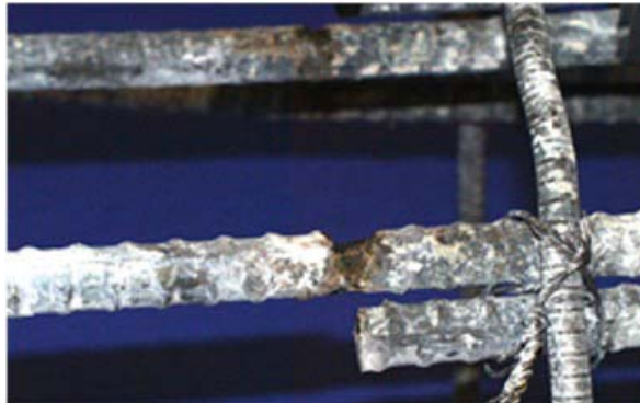
Figure 5.93 Typical corrosion and section loss found on dowels at the column-foundation interface
