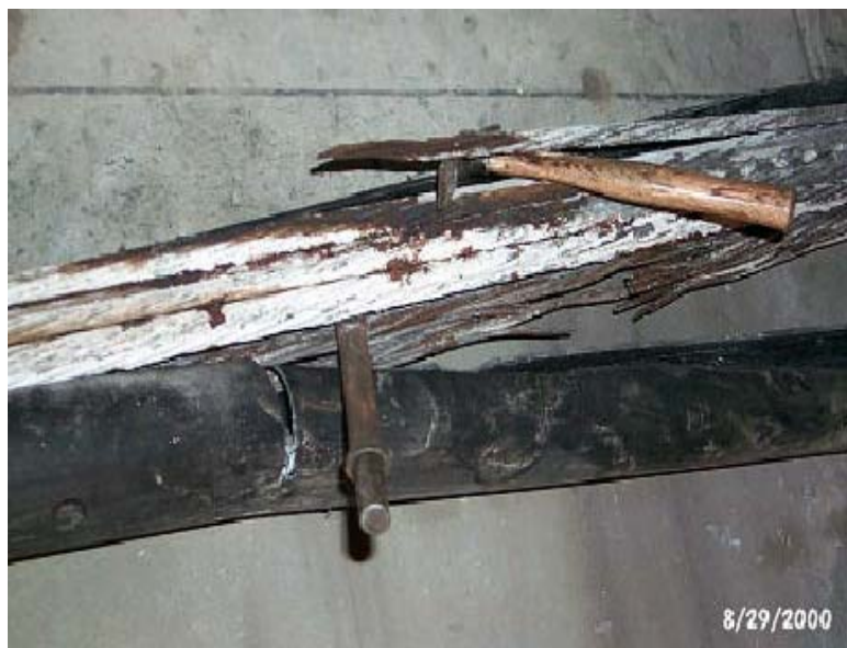
Figure 2.8 Failure of Tendon 28-6 on the Mid-Bay Bridge 2.10
