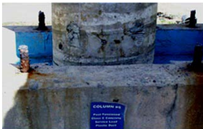
Figure 5.66 Condition of Specimen PT-TC-S-PD at the End of Testing
