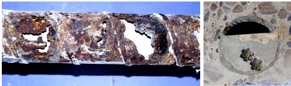
Figure 4.146 Bleed Water Void and Duct Corrosion
