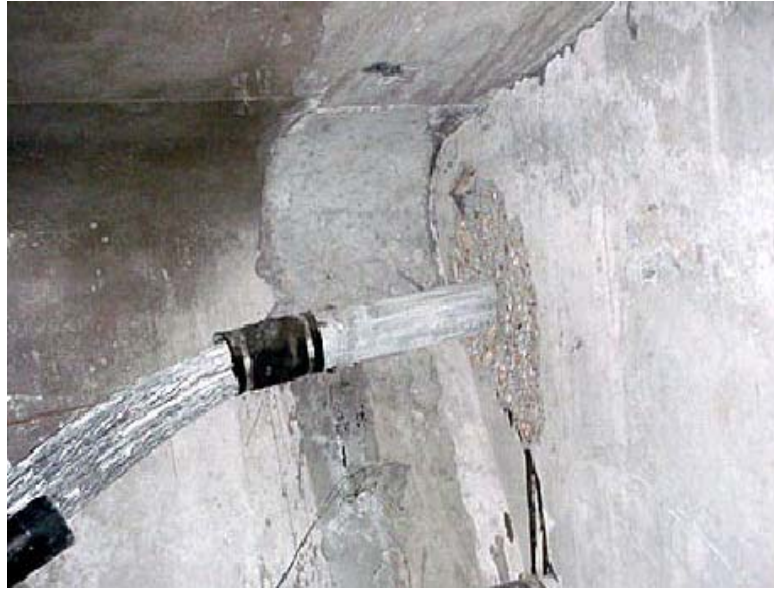
Figure 2.9 Failure of Tendon 57-1 on the Mid-Bay Bridge- At Expansion Joint Diaphragm- 2.10
