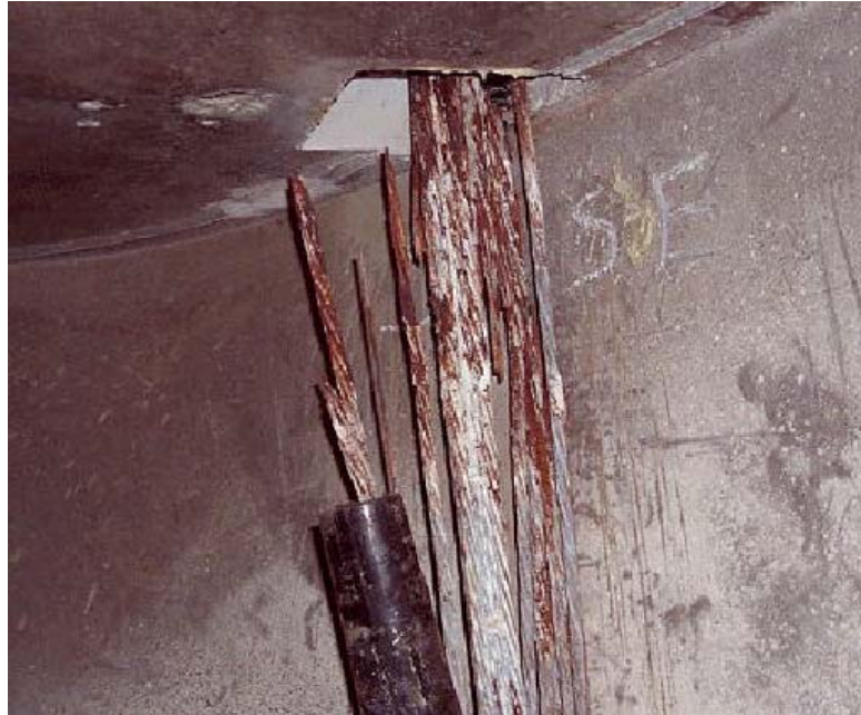
Figure 2.11 Tendon Corrosion inside the Sunshine Skyway Bridge Piers (Refer to Figure 2.3) 2.10
