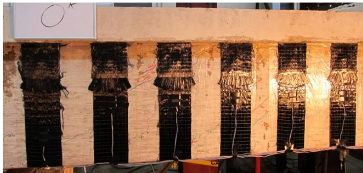
Figure 4-35 24-3-Fatigue-Fail-4 at 0-kips applied load (0-kips applied shear)
