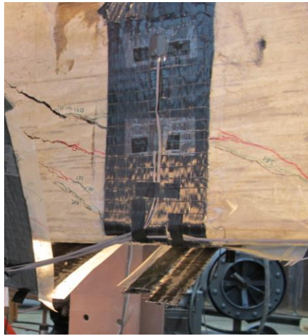
Figure 4-12 Rupture of a CFRP strip observed during 24-3-Fatigue-Fail-1
