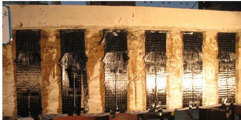
Figure 4-23 24-3-Fatigue-Fail-2 at 270-kips applied load (135-kips applied shear)
