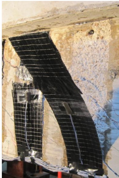
Figure 4-18 CFRP anchor failure observed during 24-3-Fatigue-Fail-2
