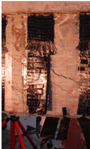
Figure 4-33 CFRP sheet rupture observed during 24-3-Fatigue-Fail-4
