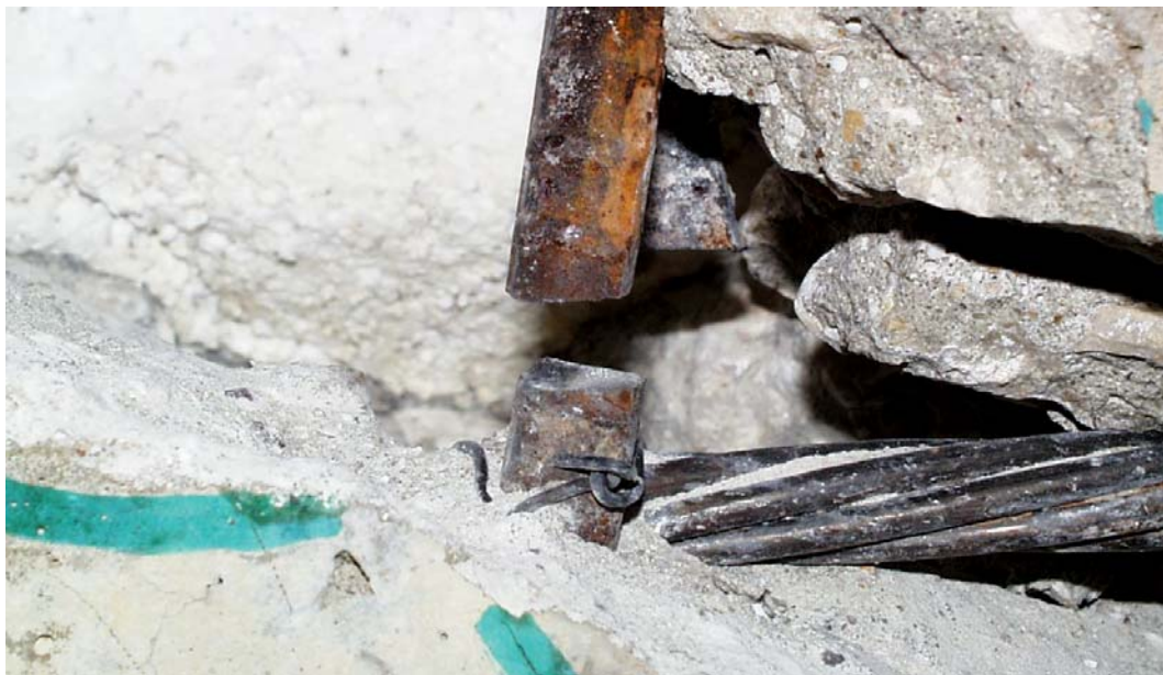
Figure 4.13 Fractured shear reinforcement (stirrup) in the east web of BG3N at failure, after removal of concrete
