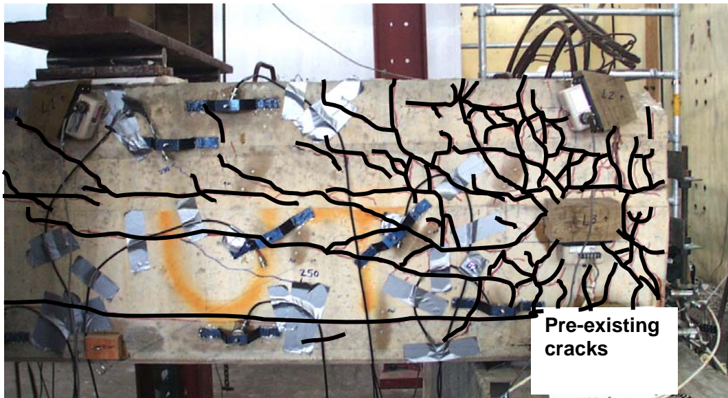
Figure 4.22 Pre-existing cracks in the west web of BG3S
