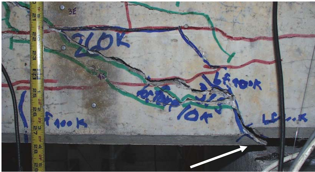
Figure 4.12 Displaced concrete section at the bottom of the east web of BG3N at failure
