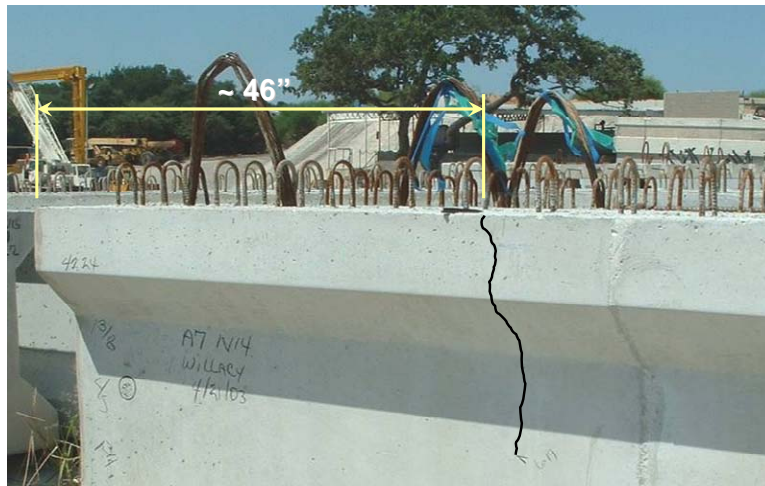
Figure 1.1 Typical flexural crack occurring at the time of release.
