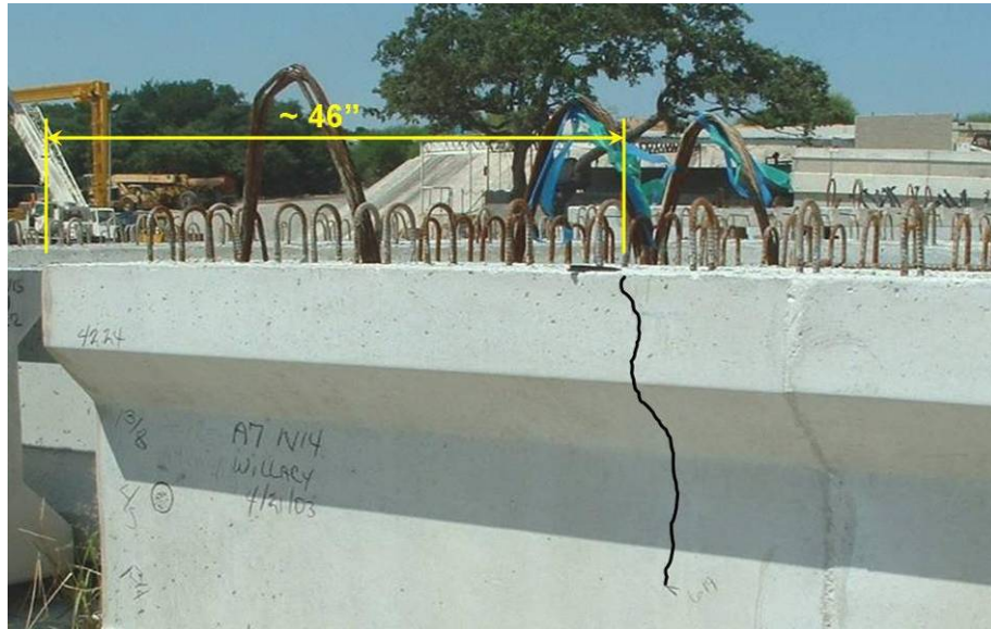
Figure 3.1 Cracking in the end of a Type IV beam, without block-out.
