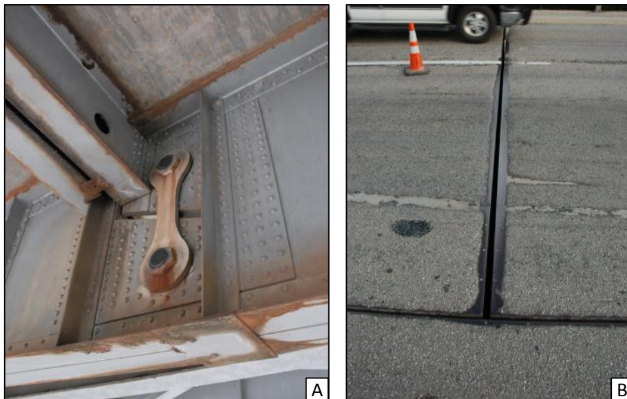
Figure 3.5 (a) Hanger detail at Medina River Bridge; (b) Road surface joint at hanger.
