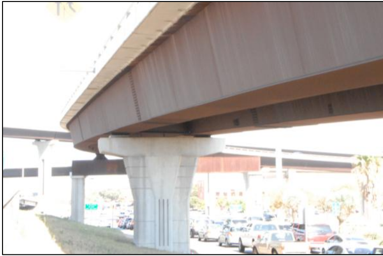
Figure 3.23 Bottom flanges of the longitudinal box girders at the US-290 Bridge bear on the piers.
