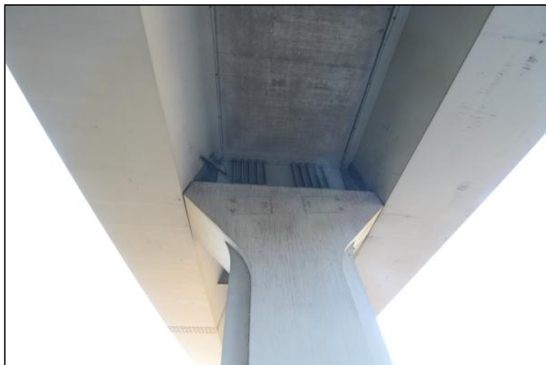
Figure 3.31 The cross beam at the I-5 Interchange Bridge bear on the piers.
