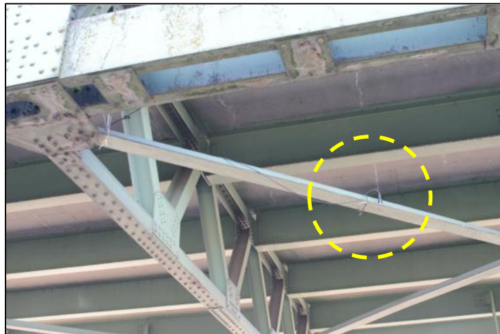
Figure 3.44 Accelerometer clamped to bottom chord brace on southbound I-5 Columbia River Bridge
