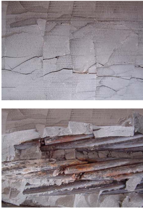
Figure 4-10: Longitudinal Cracks and Corresponding Wire Breaks
