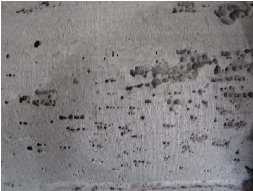
Figure 4-11: Air Voids at the Deck Anchorage – Specimen #2
