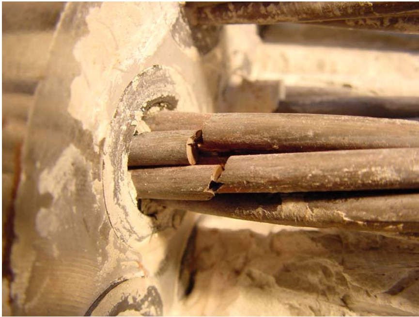
Figure 4-20: Wire Breaks – Strand #2 – Tower Anchorage – Specimen #1
