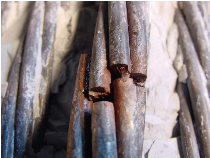
Figure 4-21: Wire Breaks – Strand #19 – Tower Anchorage – Specimen #1
