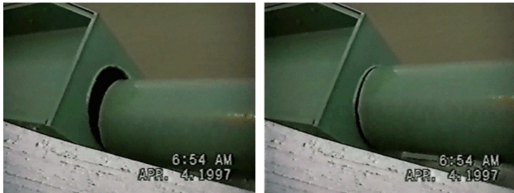
Figure 1-6: Broken Guide Pipe
