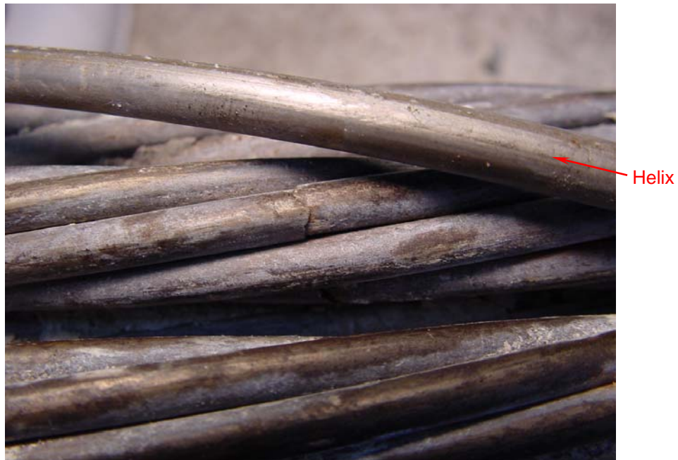
Figure 4-33: Wire Break Close to Helical Spacer – Specimen #2
