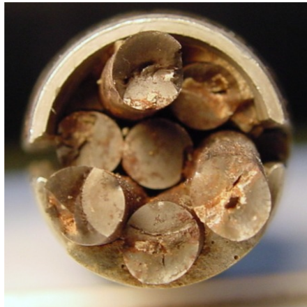
Figure 4-32: Fracture Surfaces – Strand #2 – Tower Anchorage – Specimen #2
