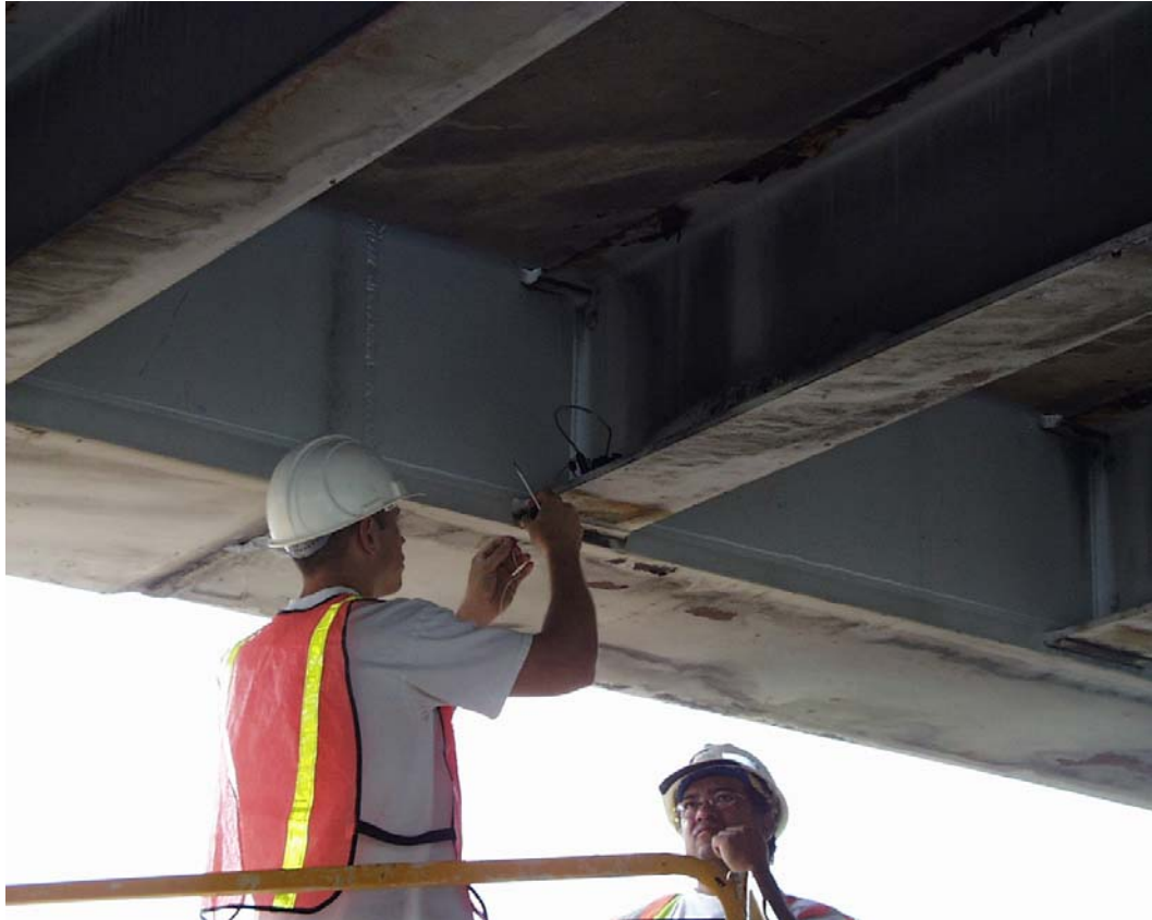
Figure 3-12: MicroSAFE Unit Installation
