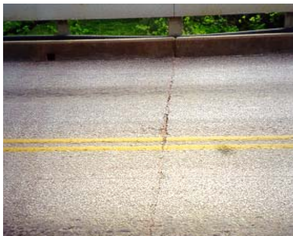
Figure 4.17 Cracked Slab over Floor Beam
