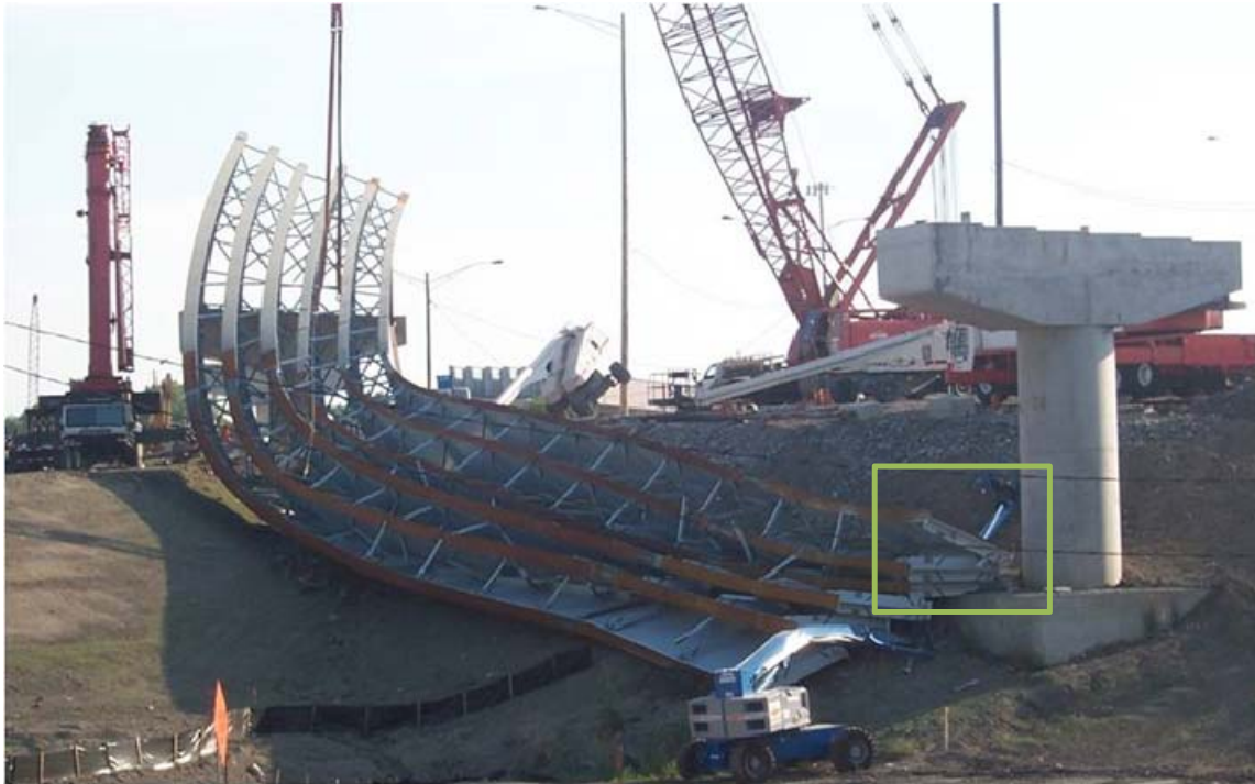
Figure 1.1: Curved Bridge Collapse [Photo Courtesy ILDOT]
