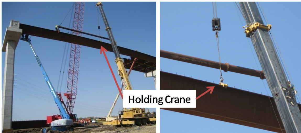
Figure 4.3: Holding Crane and its Attachment to the Top Flange of a Girder
