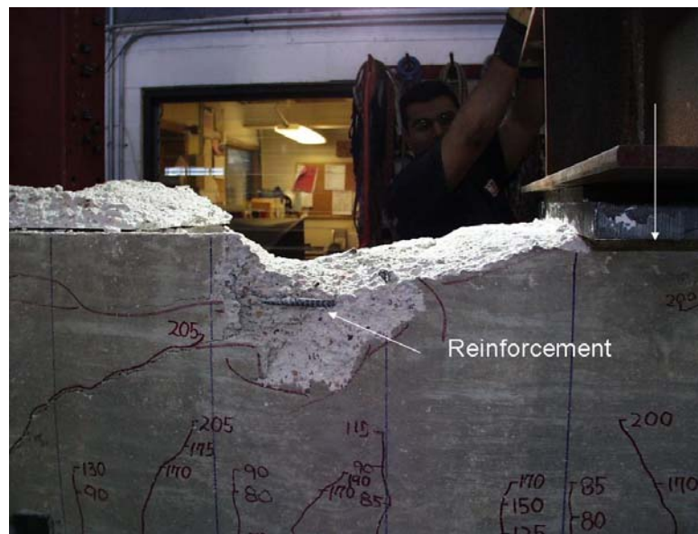
Figure 3.12 Picture of the failure zone after removal of loose concrete
