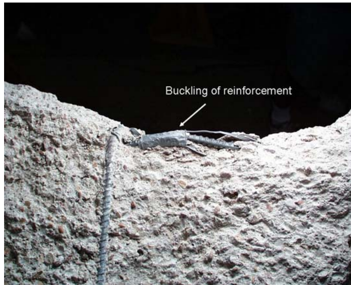
Figure 3.13 Buckling of compression reinforcement
