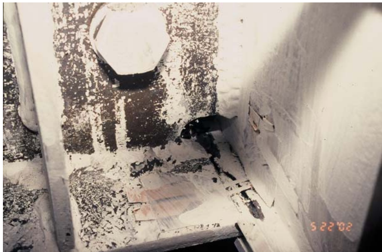
Figure 4.24 Point Switch Bridging 1/10-in. Wide Crack
