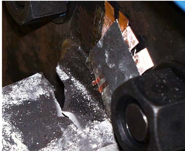
Figure 4.16 Photograph of Mill Scale Residue on Adhesive Pad on Top Flange
