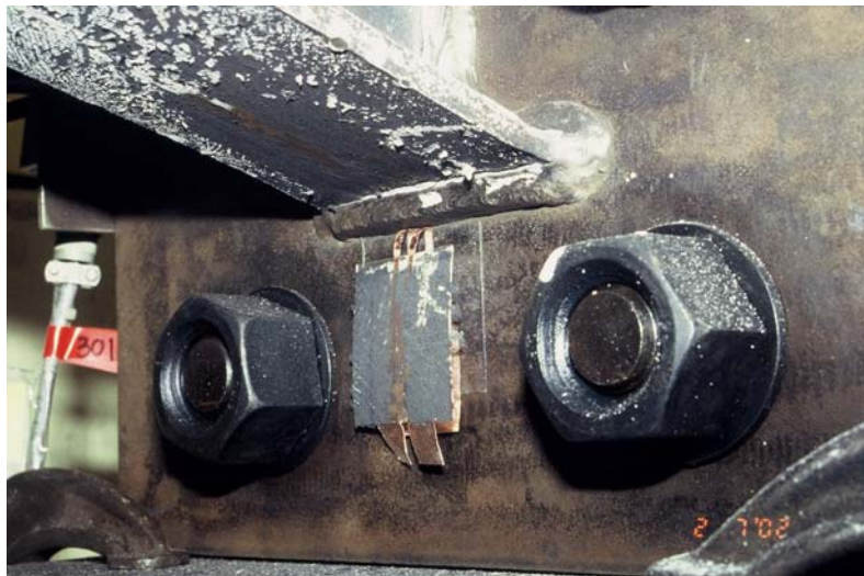
Figure 4.17 Photograph of Mill Scale Residue on Adhesive Pad on Bottom Flange
