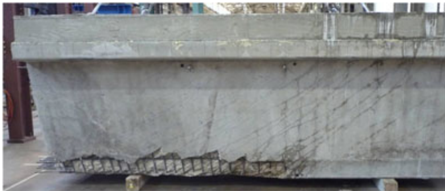
(e) Horizontal shear failure (Adopted from Hovell, et al. 2010)
