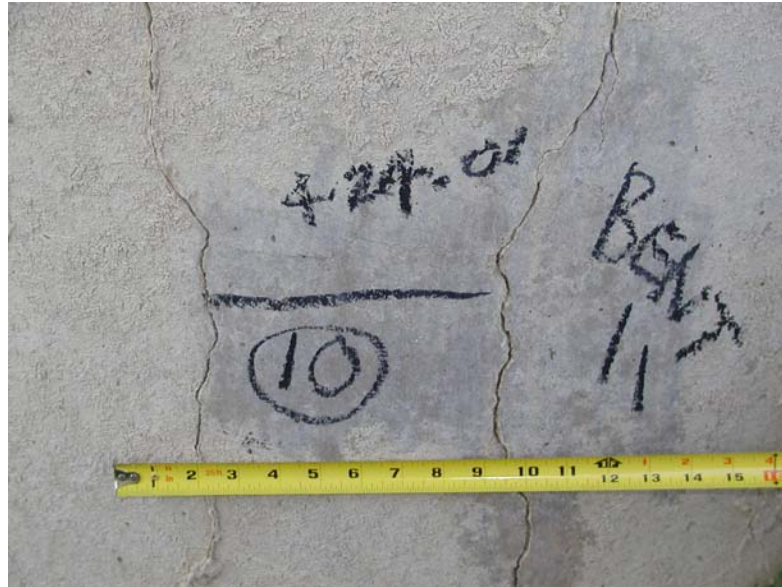
Figure 7.49: Column cracking at Point 10 near waterline, Bent 11 (10/15/01)
