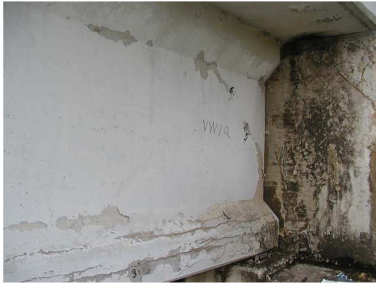
Figure 7.12: Cracks at end of NW Girder 1, US-90 (6/22/01)
