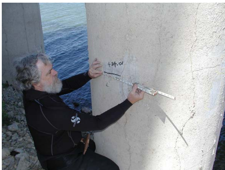
Figure 7.45: Example of column cracking near waterline of Bent 11 (Point 10) (4/24/01)
