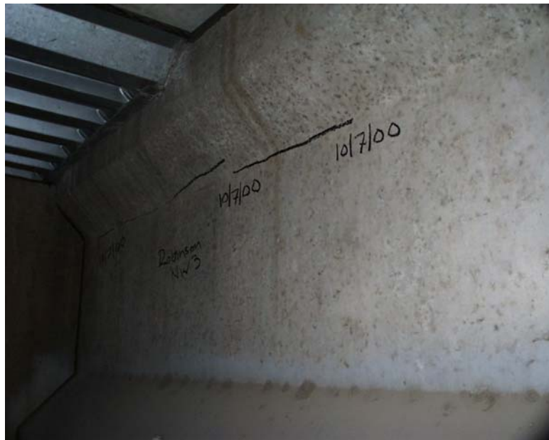
Figure 7.16: Extension of new cracking on south face of NW Girder 3, Robinson Road (10/7/00)
