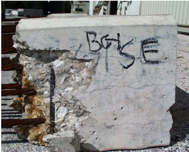
Figure 3.12: Cracking on left face of Slice BG1S
