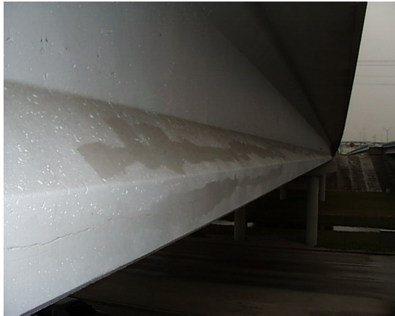
Figure 7.31: Sealed cracks along girder flange near Point 6, Beltway 8 structure (12/11/01)
