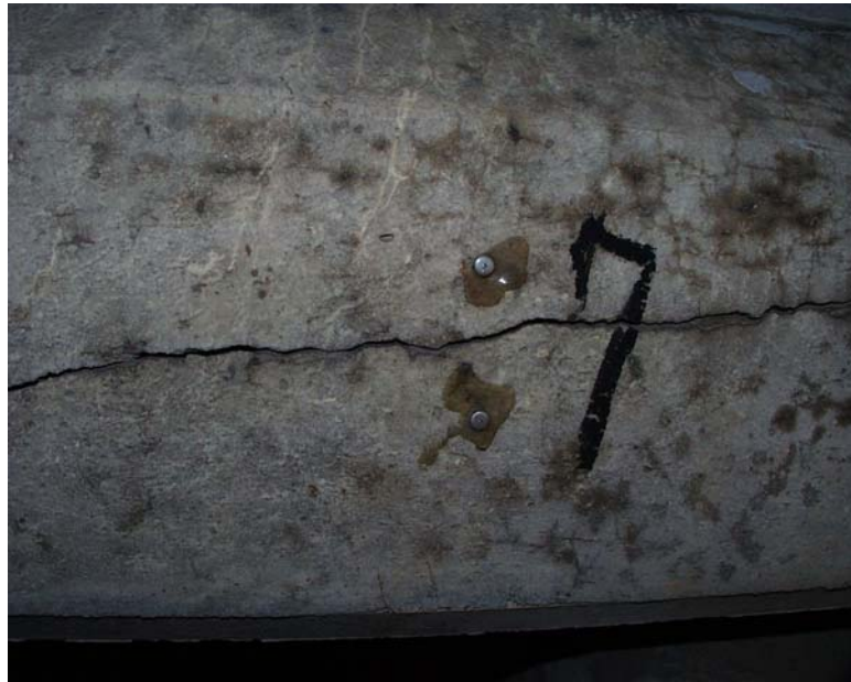
Figure 6.13: One set of Demec discs for monitoring crack width
