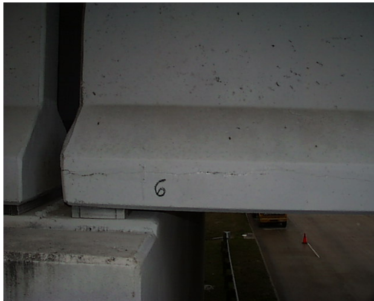
Figure 7.30: Cracking near Point 6, Beltway 8 structure (12/11/01)
