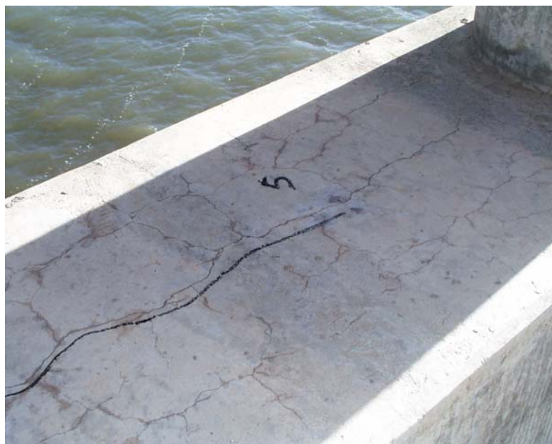
Figure 7.40: Map cracking on tie beam, Bent 5 (12/18/00)
