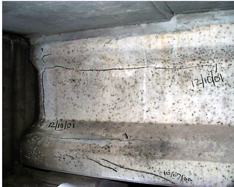
Figure 7.7: New cracks on south face of SW Girder 3 at west abutment, I-10 (12/10/01)
