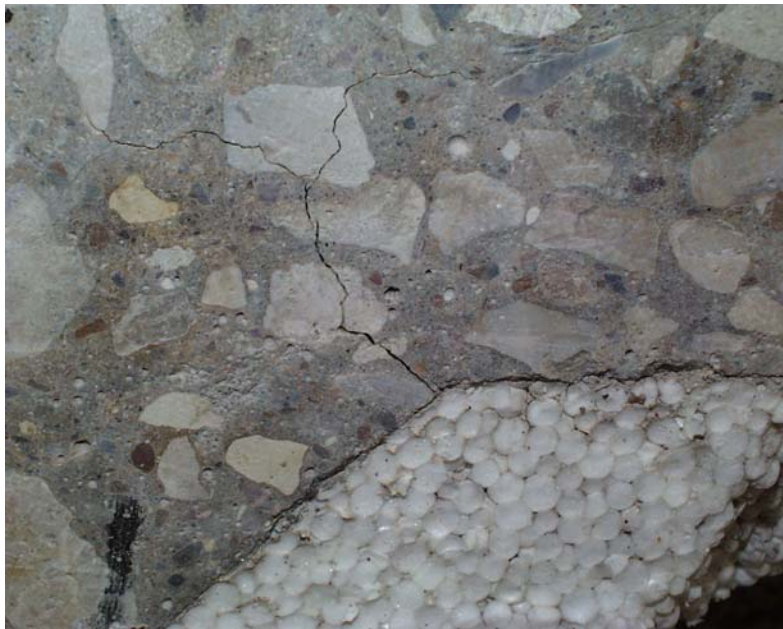
Figure 3.13: Cracks at left inner corner of Slice BG1S
