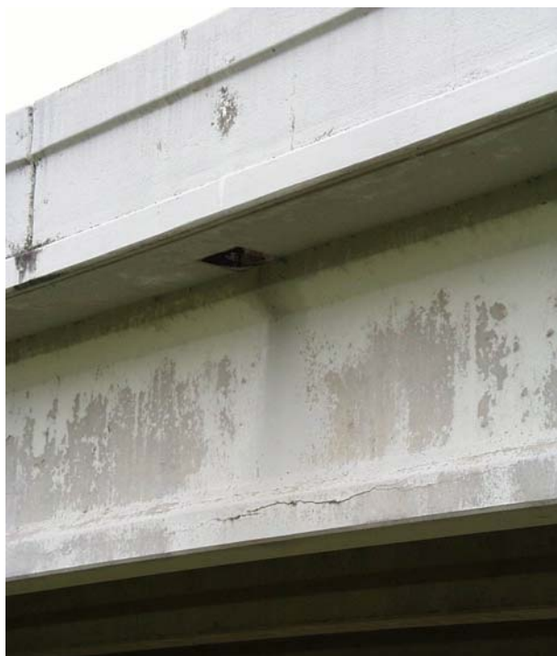
Figure 7.10: Typical crack under drain at US-90 structure (10/6/00)
