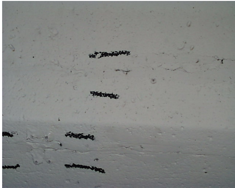
Figure 7.13: Close-up view of Point 10 (bottom, left pair of Demec discs) and Point 8 (top), US-90 (12/11/01)
