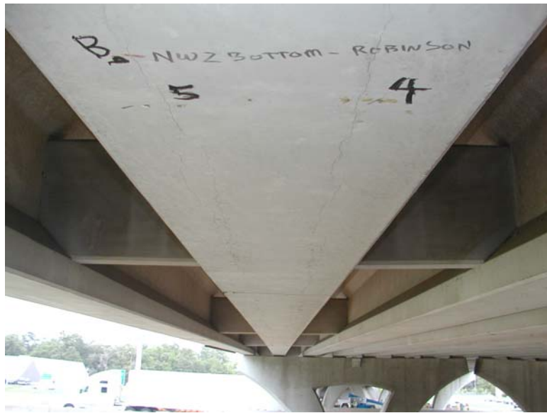
Figure 7.18: Extension of cracking on underside of NW Girder 2, Robinson Road (6/21/01)
