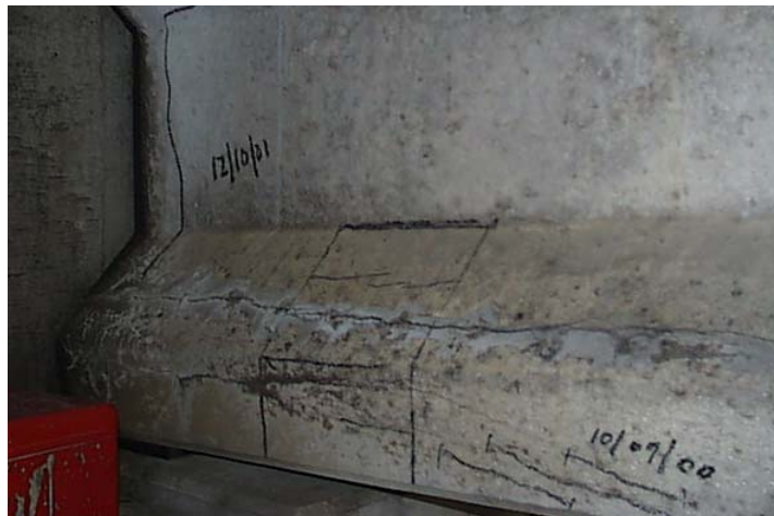
Figure 6.15: Representative areas used for crack ratios, I-10 structure
