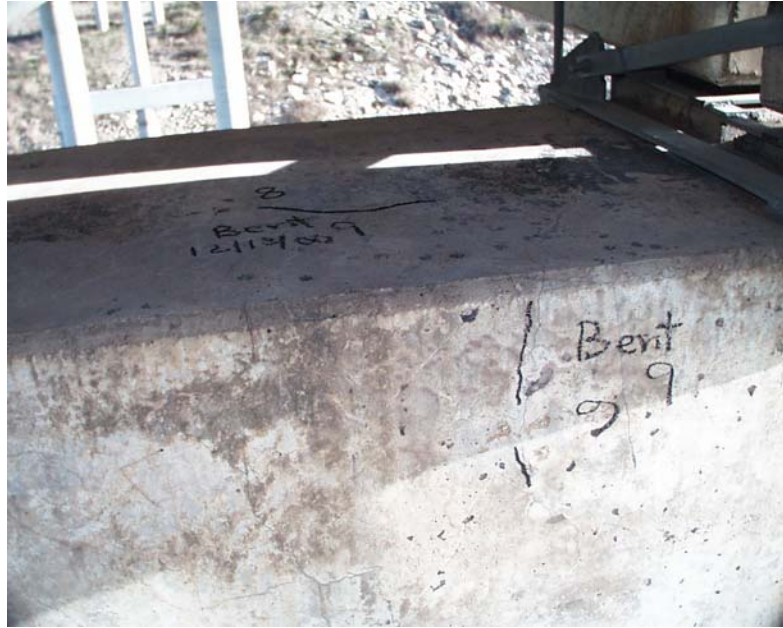
Figure 7.41: Cracking on bent cap, Bent 9 (12/18/00)
