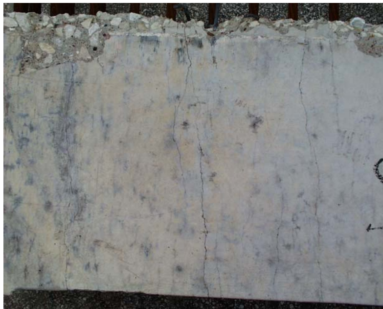
Figure 3.21: Cracking on bottom face of Slice BG4S2
