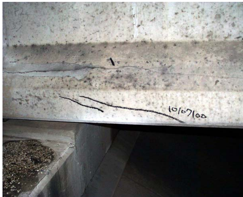
Figure 7.3: New diagonal cracks on I-10 SW Girder 4, Face 5 (10/7/00)
