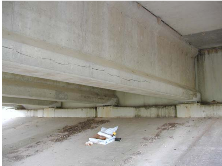
Figure 7.11: Extension of existing cracking on north surface (Face 5) of NW Girder 2, US-90 (6/22/01)
