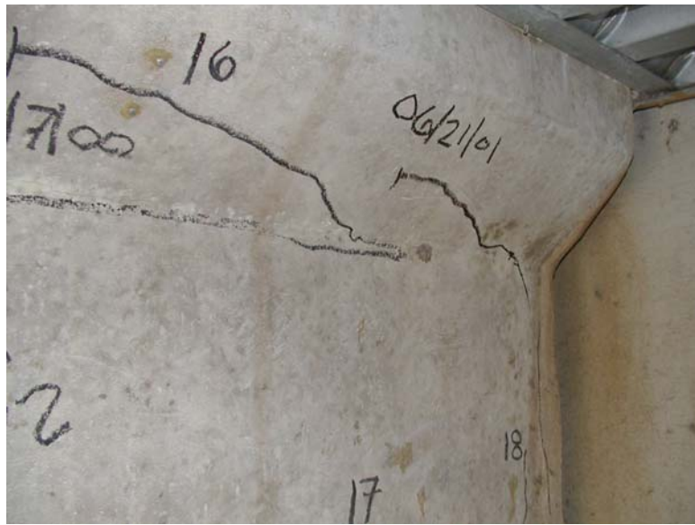
Figure 7.17: Extension of cracking on NW Girder 2, Robinson Road (6/21/01)
