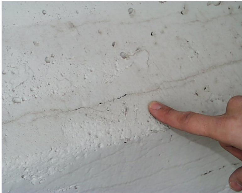
Figure 7.14: Apparent cracking through sealant, US-90 (12/11/01)
