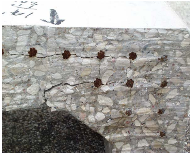
Figure 3.20: Cracking in back face of Slice BG4S2
