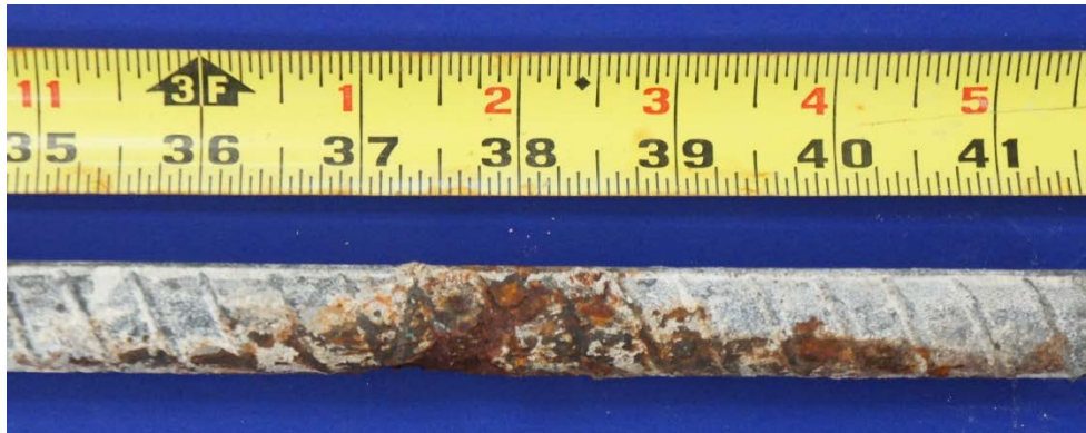
Figure 6.166: Appreciable Cross Sectional Area Loss due to Pitting on the South Coated Longitudinal Bar from Specimen 7.4
