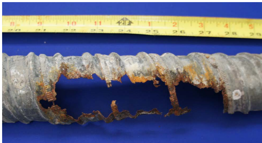
Figure 6.76: Hole on the Top at Midspan of the North Duct from Specimen 4.1
