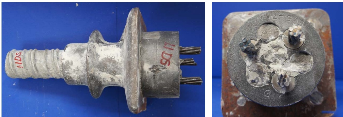
Figure 6.21: Dead End South Side Anchorage Assembly (Left) and Exposed Face of Anchor Head and Anchorage Plate (Right) from Specimen 1.1
