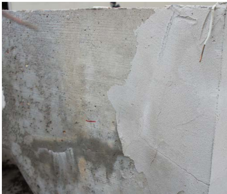
Figure 6.59: Efflorescence from Re-entrant Crack on North side of Specimen 3.3 Live End
