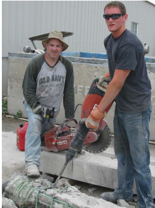
Figure 6.5: Chipping Post-Tensioning Components and Mild Reinforcement from Specimen Blocks (Kevin Moyer on the left and Michael Weyenberg on the right)
