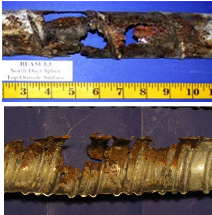
Figure 7.29: Typical Galvanized Steel Duct from Project 0-1405 5 (Top) and Project 0-4562 (Bottom)
