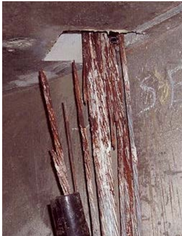
Figure 1.3: Tendon Corrosion in the Sunshine Skyway Bridge Piers 33
