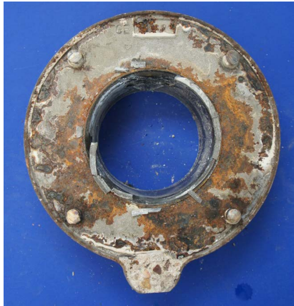
Figure 6.161: Corrosion on Exposed Face of Dead End Anchorage Plate from Specimen 7.3
