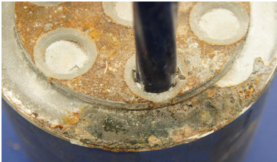
Figure 6.174: Moderate Corrosion on Unexposed Face of the Dead End Anchor Head from Specimen 7.4
