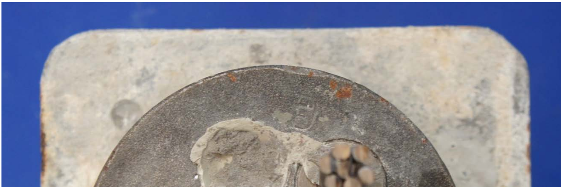
Figure 6.45: Light Surface Corrosion of Exposed Face of North Anchor Head from Specimen 1.4
