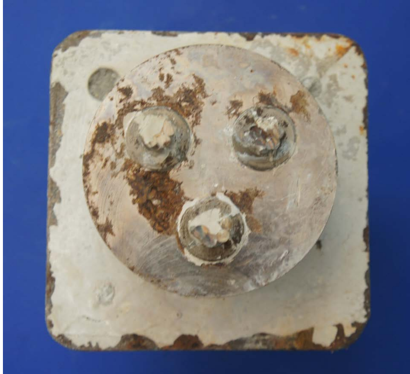
Figure 6.125: Exposed Faces of Live End South Anchorage Plate and Anchor Head from Specimen 5.3
