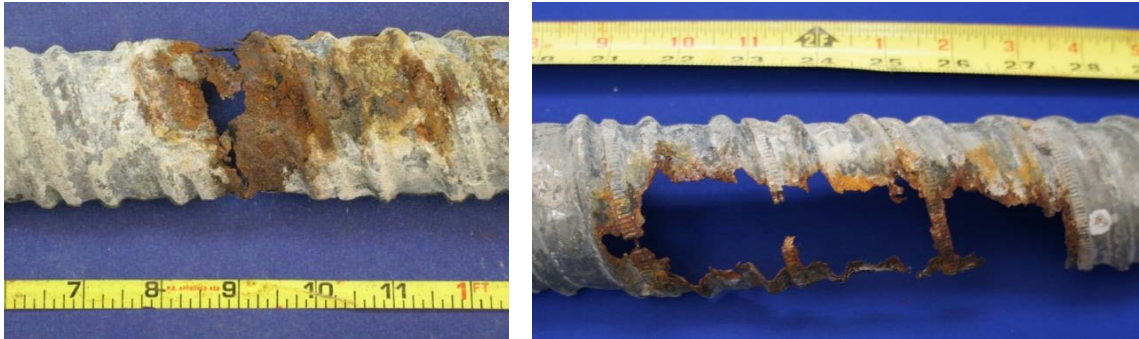
Figure 7.22: Typical Galvanized Duct from 4 year 2 (Right) and 6 Year (Left) Autopsy Periods
