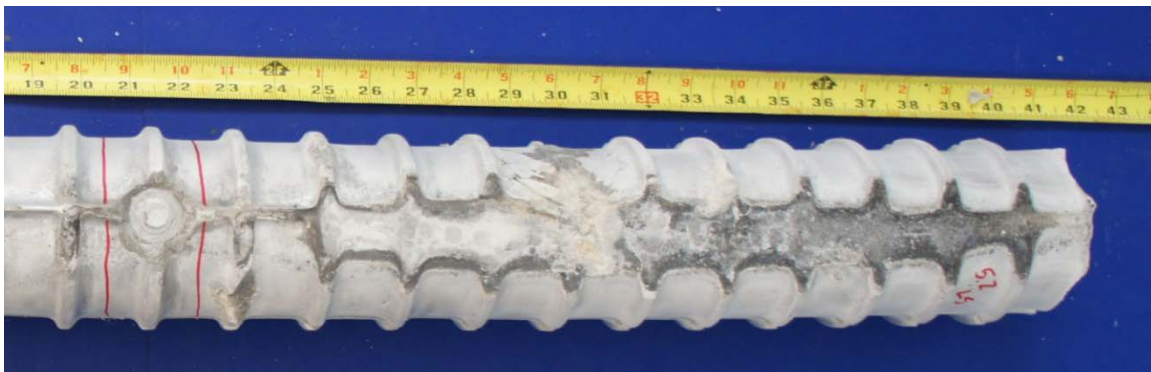
Figure 6.111: Large Void in Grout on Top Live End Side of South Tendon from Specimen 5.2
