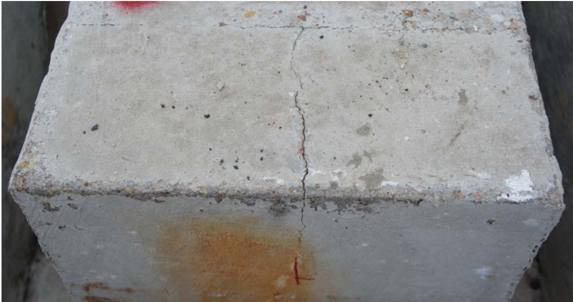
Figure 6.149: Crack at Interface of the Backfill Mortar and Base Concrete at the Live End of Specimen 7.3
