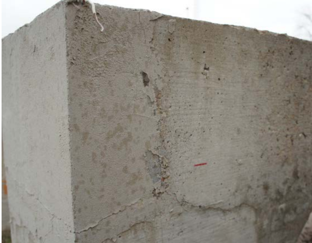
Figure 6.37: Separation of the Backfill Mortar of the Live End Anchorage Pocket from the Base Concrete of Specimen 1.4
