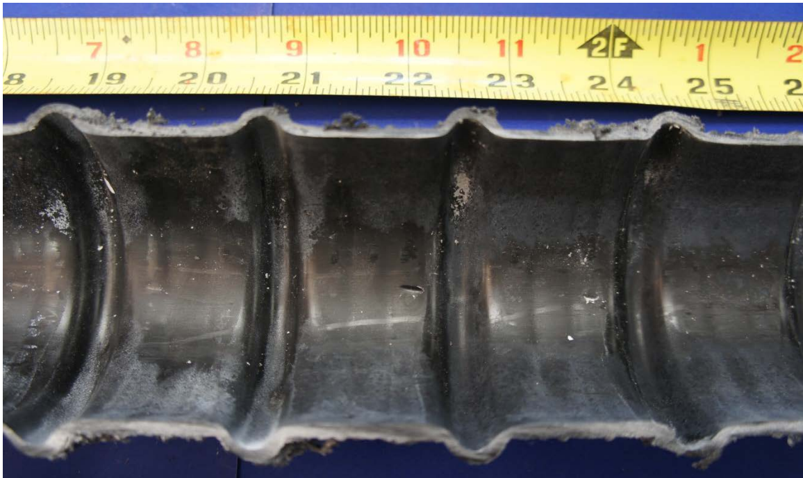
Figure 6.168: Gouge on the Bottom Inner Surface of the Duct from Specimen 7.4
