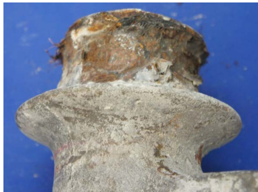
Figure 6.55: Moderate Surface at South Dead End Interface of Duct and Anchorage Plate of Specimen 2.3
