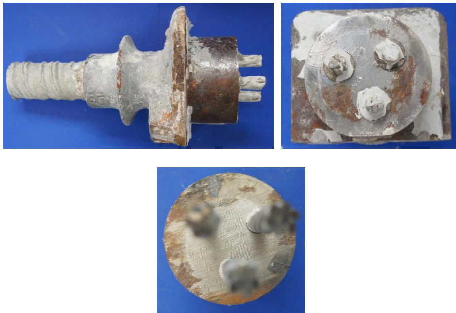
Figure 6.33: Light Surface Corrosion on Anchorage Components: Bottom of Anchorage (Top Left), Exposed Surface of Anchorage Plate and Head (Top Right), and Unexposed Surface of Anchor Head (Bottom) of Specimen 1.3
