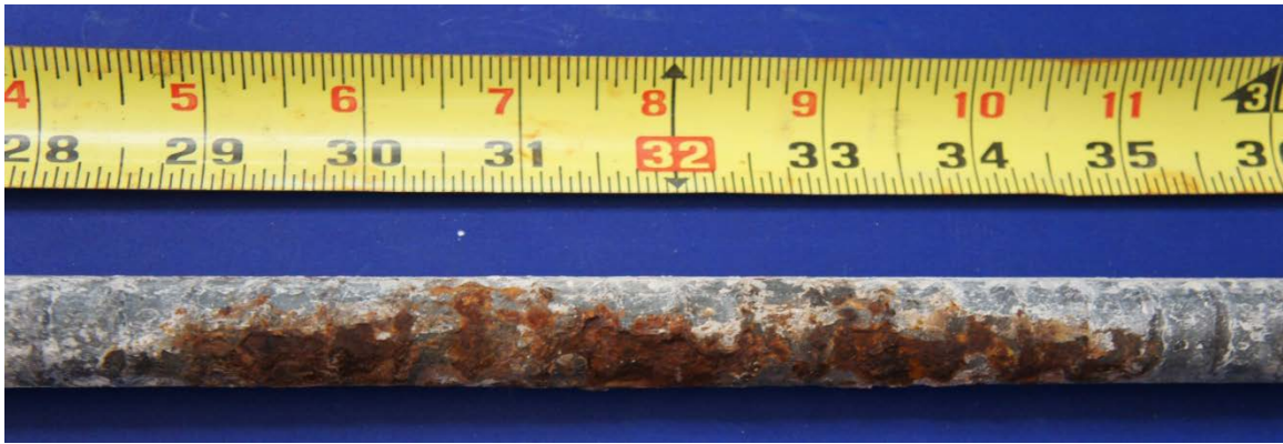
Figure 6.153: Pitting on North Longitudinal Uncoated Bar from Specimen 7.3
