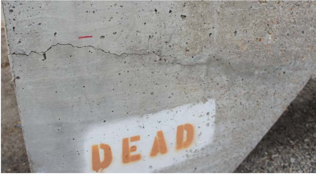
Figure 6.26: Crack at the Re-Entrant Corbel Corner on the North Side of the Dead End of Specimen 1.3
