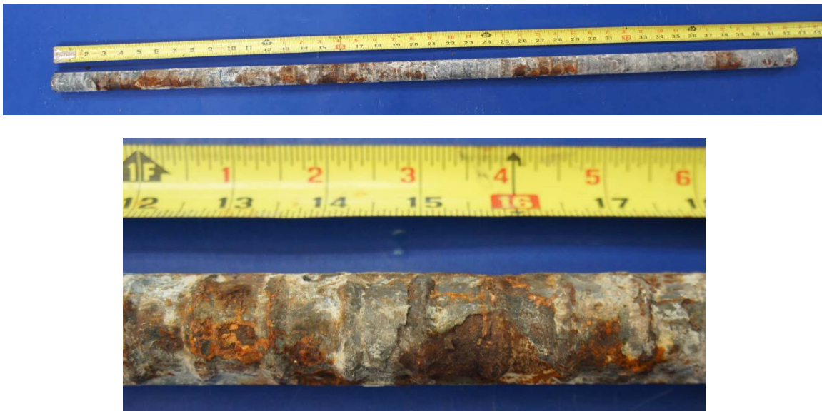
Figure 6.94: Moderate and Light Corrosion (Top) and Pitting (Bottom) on South #8 Uncoated Bar from Specimen 4.4
