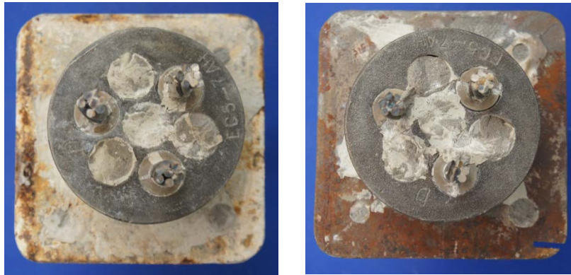
Figure 7.11: Corrosion on Exposed Faces of Galvanized (Left) and Non-Galvanized (Right) Anchorage Plates
