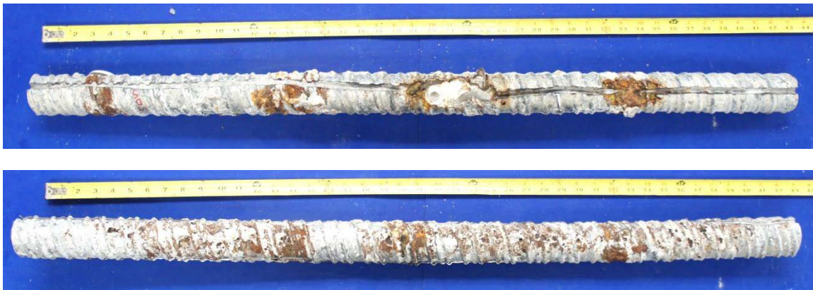
Figure 6.41: Specimen 1.4 Top of North Duct (Top) and Bottom of South Duct (Bottom)
