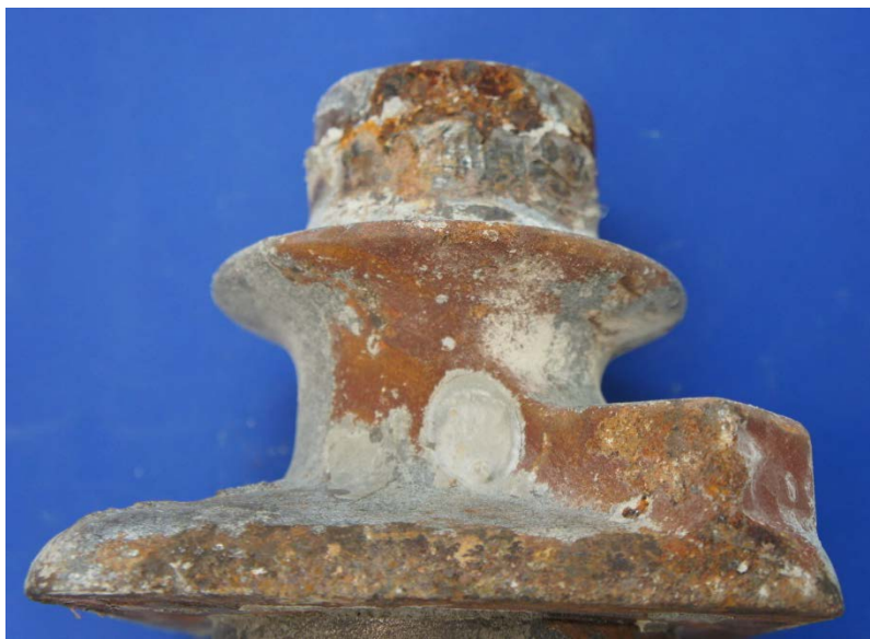
Figure 6.68: Light Surface Corrosion on Bottom of the North Dead End Anchorage Plate from Specimen 3.3
