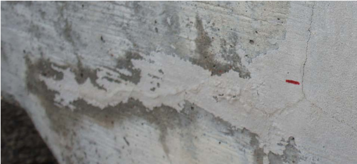
Figure 6.72: Moisture Observed around the Edge of North Live End Re-entrant Corbel Corner Crack of Specimen 4.1
