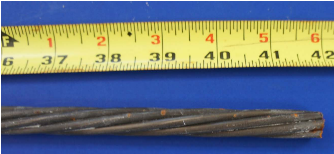
Figure 6.102: Light Corrosion on a North Strand from Specimen 5.1
