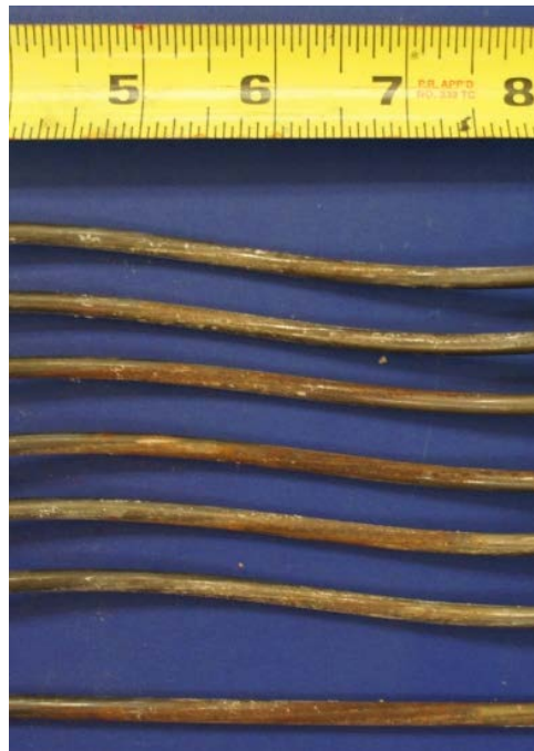
Figure 6.56: Mild Pitting on Inner and Outer Wires of a Strand from the Dead End Anchorage Region of Specimen 2.3
