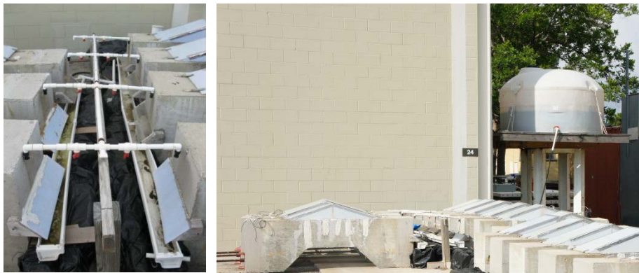
Figure 4.2: Spray System 2 (Left) and Bulk Storage Tank (Right)
