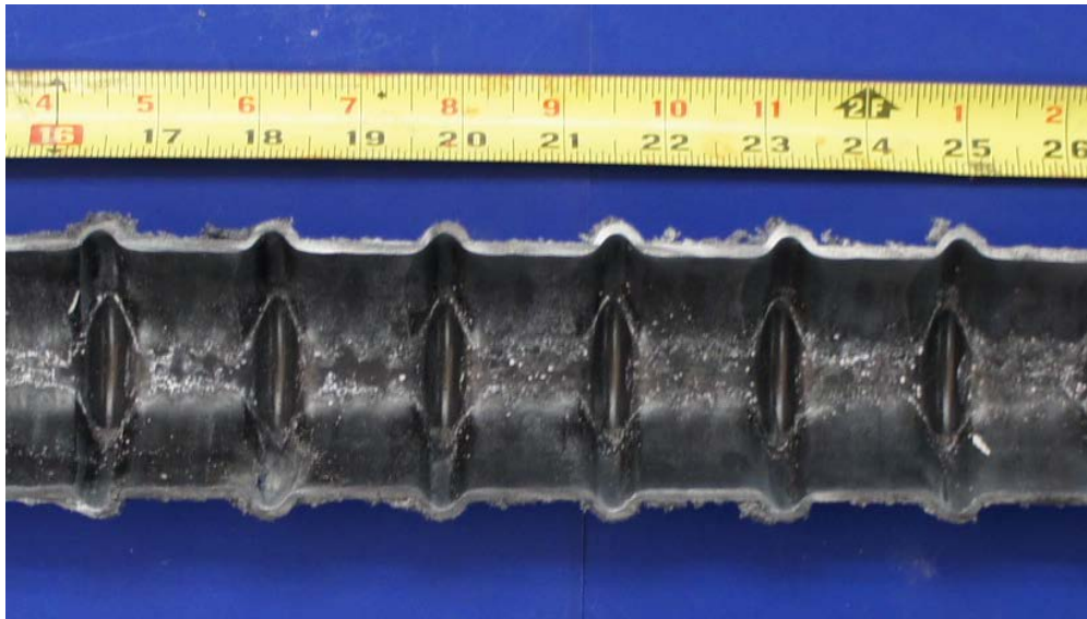
Figure 6.155: Indications of Voids in Grout on Top Surface of Duct from Specimen 7.3
