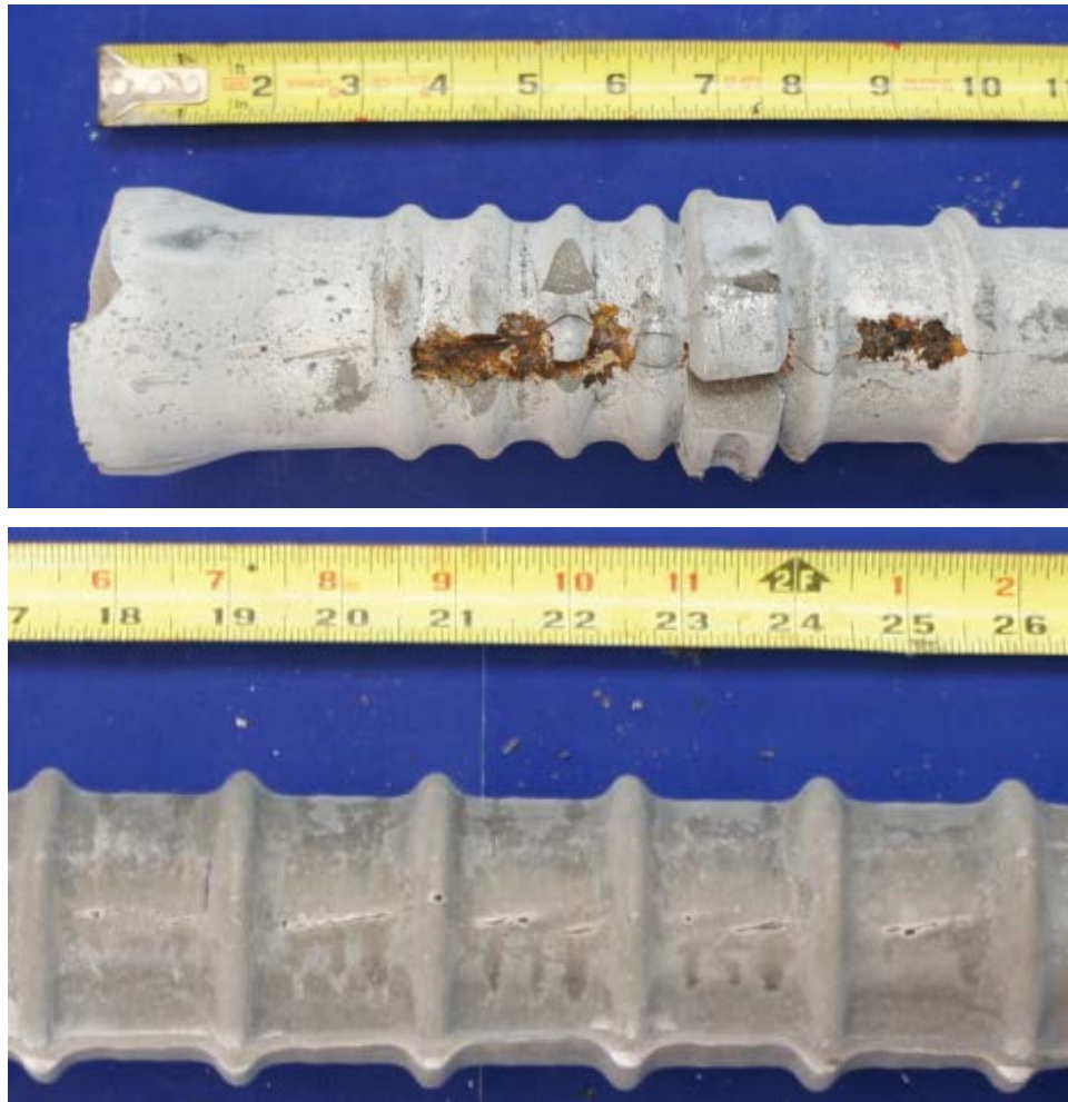
Figure 6.135: Rust Stain and Longitudinal Cracking at the Dead End Grout Vent (Left) and Visible Wires on the bottom of the Grout (Right) of Specimen 7.2
