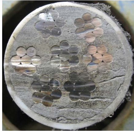
Figure 4.9: Tendon Cross Section - Specimen 3 (near south anchor end)
