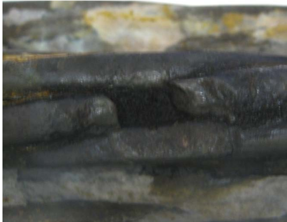
(c) Wire Fracture
