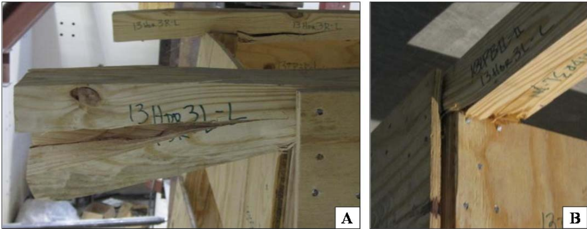
Figure 5.85 Condition of the Headers A) Split Left Header (foreground) and Split Right Header (background) B) Bearing of Left Front Post into Left Header
