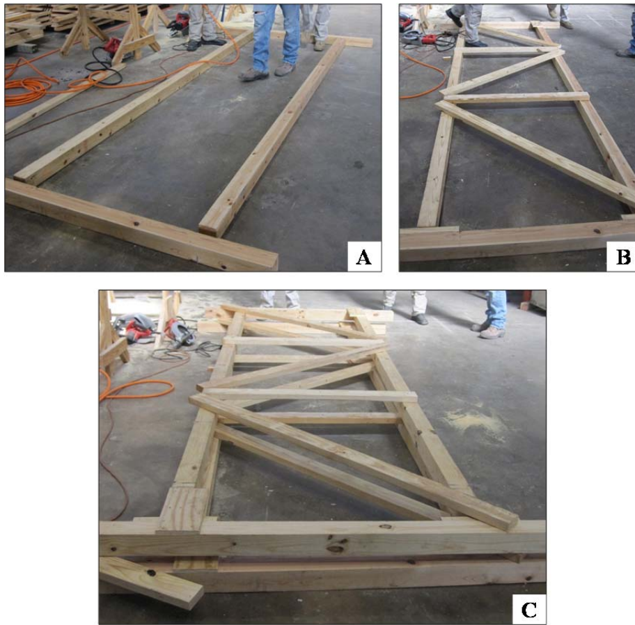
Figure 4.14 Fabrication of LP Photographs A) Layout of Main Elements B) Layout of Braces C) Using the First Side as a Guide for the Assembly of the Second Side
