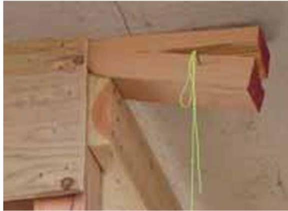
Figure 2.11 Split Header Due to Overload, ( FEMA StS2 Summary- Testing of Laced Post & Plywood Laced Posts, 2011 )
