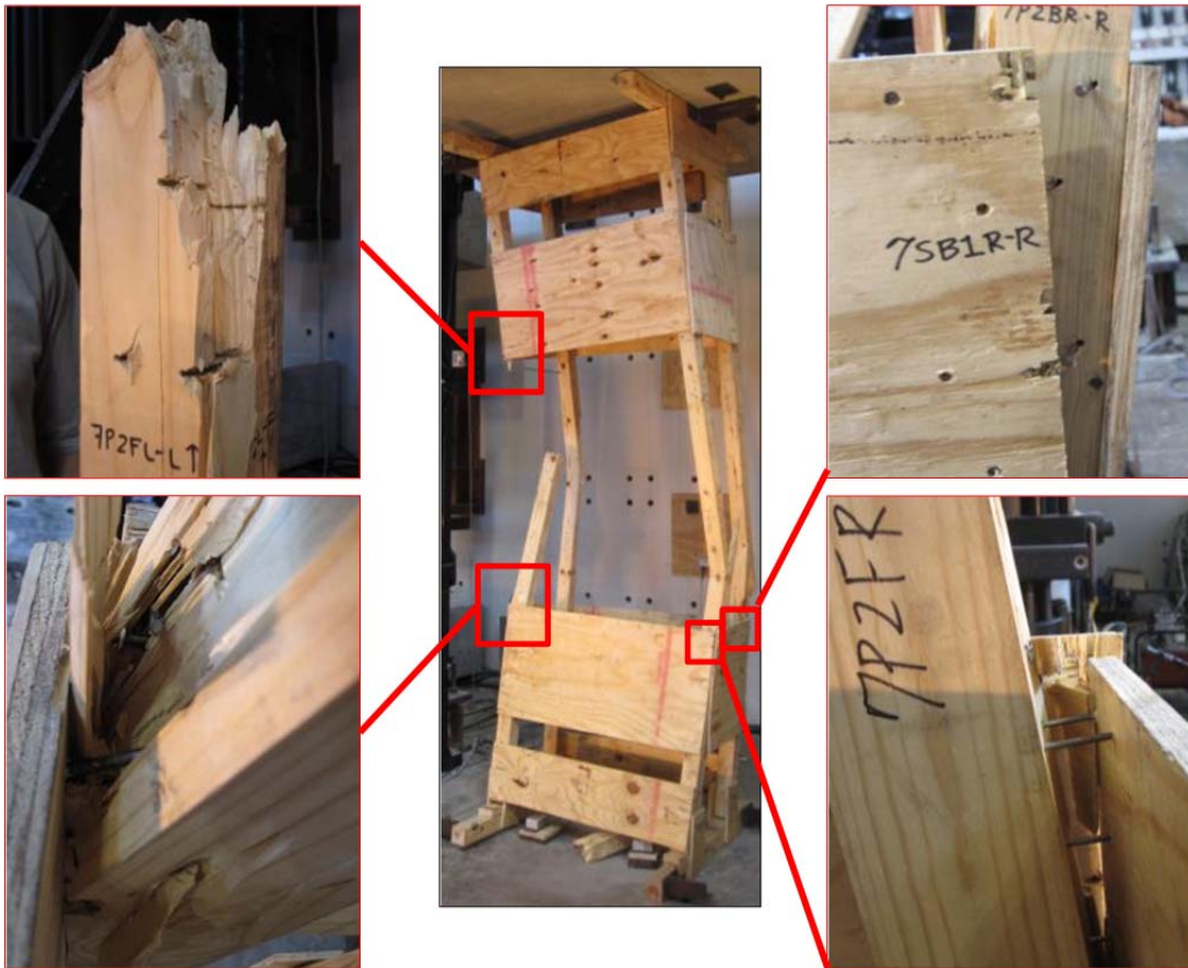
Figure 5.45 Regions of Significant Brace Connection Failures
