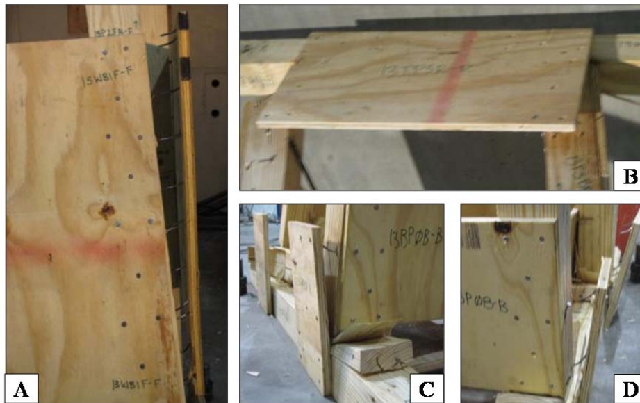
Figure 5.84 Brace Failures A) 1 st Level Brace on Right Side B) Top Plate on Right Side C) Gusset Plates on Right Side D) Gusset Plates on Left Side
