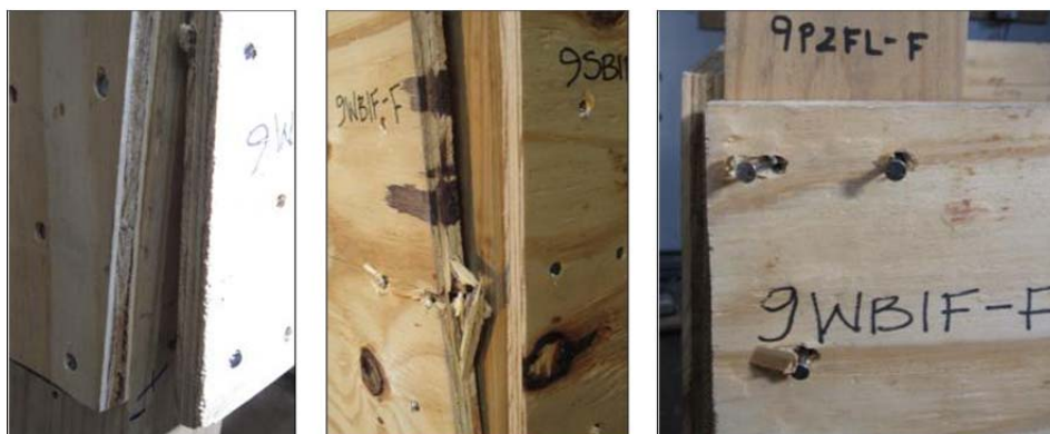
Figure 5.59 Photographs of Brace Connection Failures
