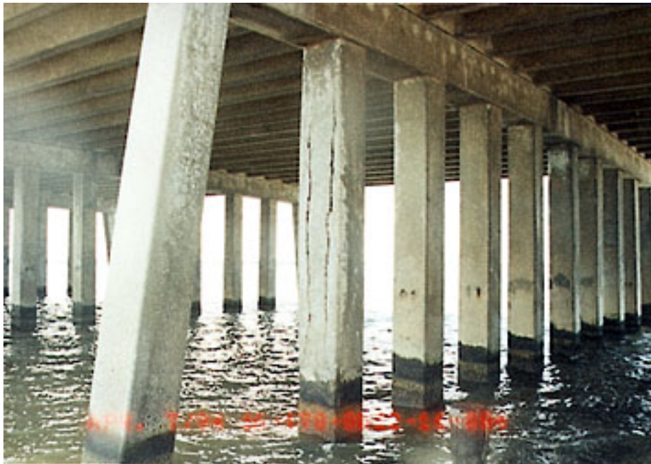
Figure 2.9: Face Splitting of a Bridge Column in Corpus Christi
