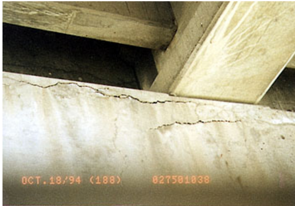
Figure 2.4: Top and Side Splitting of Upper Reinforcement in Bent Cap (Amarillo)
