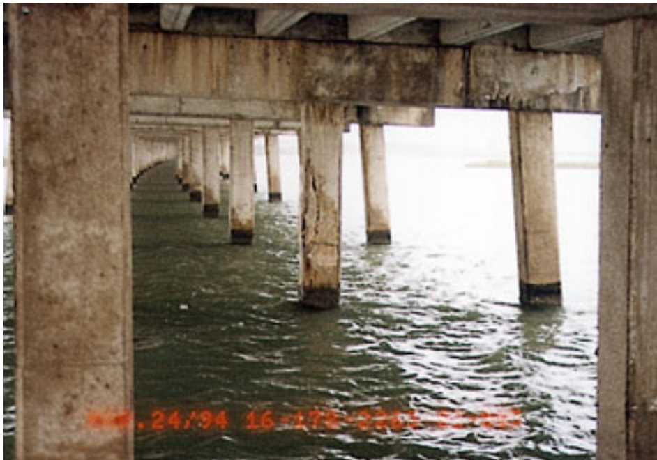
Figure 2.8: Horizontal Splitting of the Upper and Lower Reinforcement in a Typical Bent Cap
