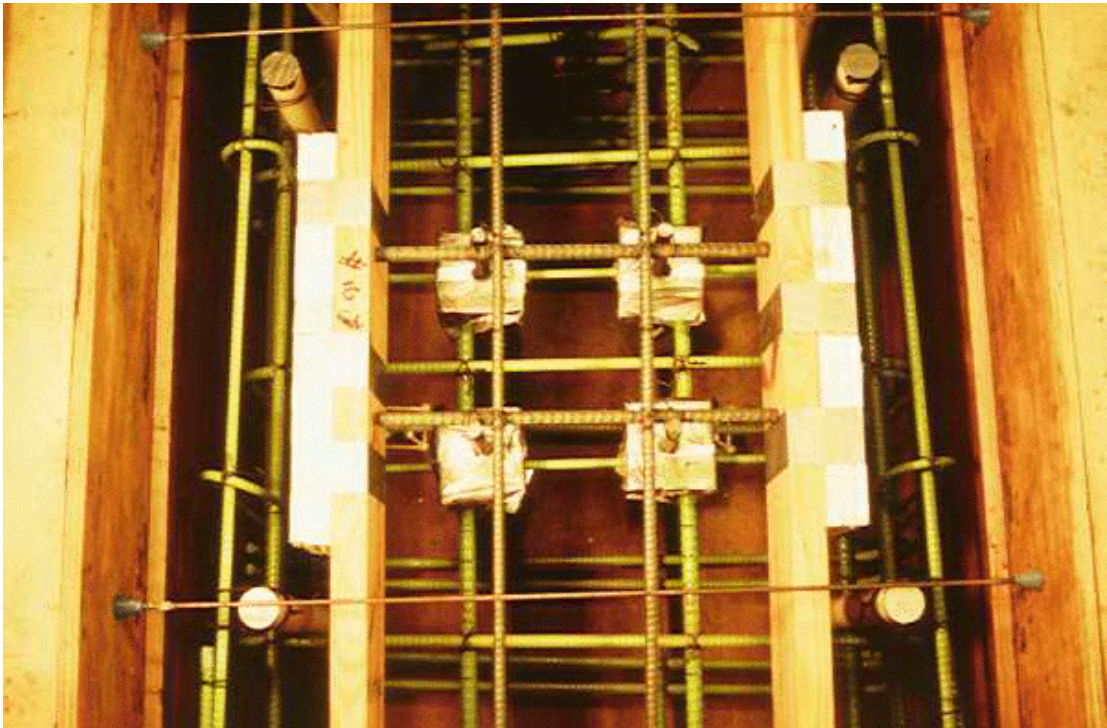
Figure 3.11: The Pipe Sleeves for the Service Load Post-Tensioning Bars Prior to Casting
