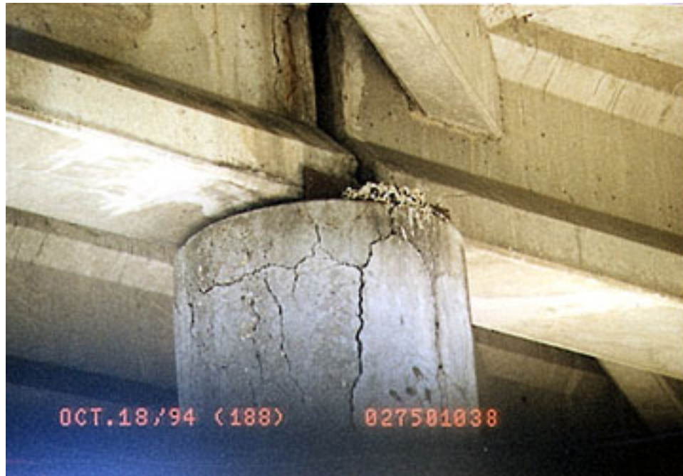
Figure 2.6: Single Column Directly under a Construction Joint in Amarillo.
