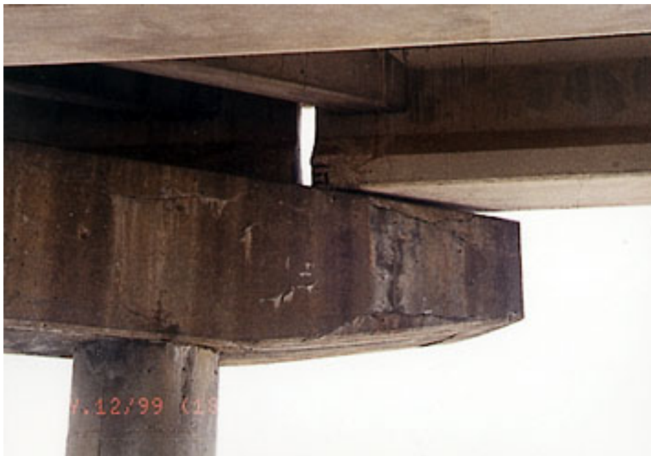
Figure 2.5: Severe Deterioration of an Amarillo Bent Cap
