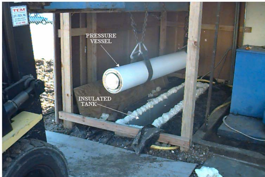
Figure 5-15: Sealed Pressure Vessel being Placed in Insulated Tank
