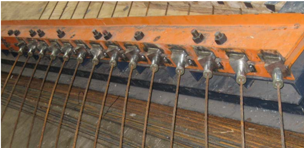
Figure 5.8: Live end anchorage after stressing strands for P45P60-1 (similar to dead end)
