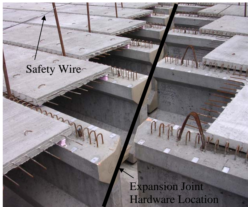
Figure 1.6: Complex geometry and hazardous work environment at an unfinished skewed expansion joint (Agnew 2007)
