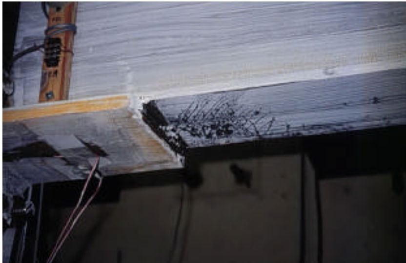
Figure 6.4 – Specimen 2 Beam Yield Pattern at 2.0% Drift
