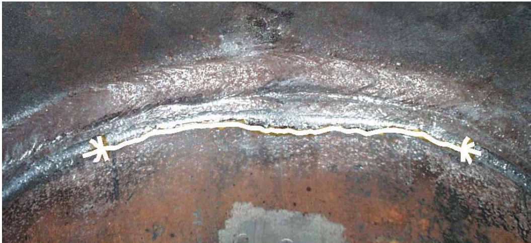
Figure 7.14 Failure of UIT Treated Socket Connection Specimen – Painted line indicates extent of visible cracking.
