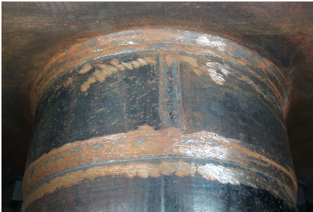
Figure 7.27 Failure of Externally Stiffened Collar Specimen
