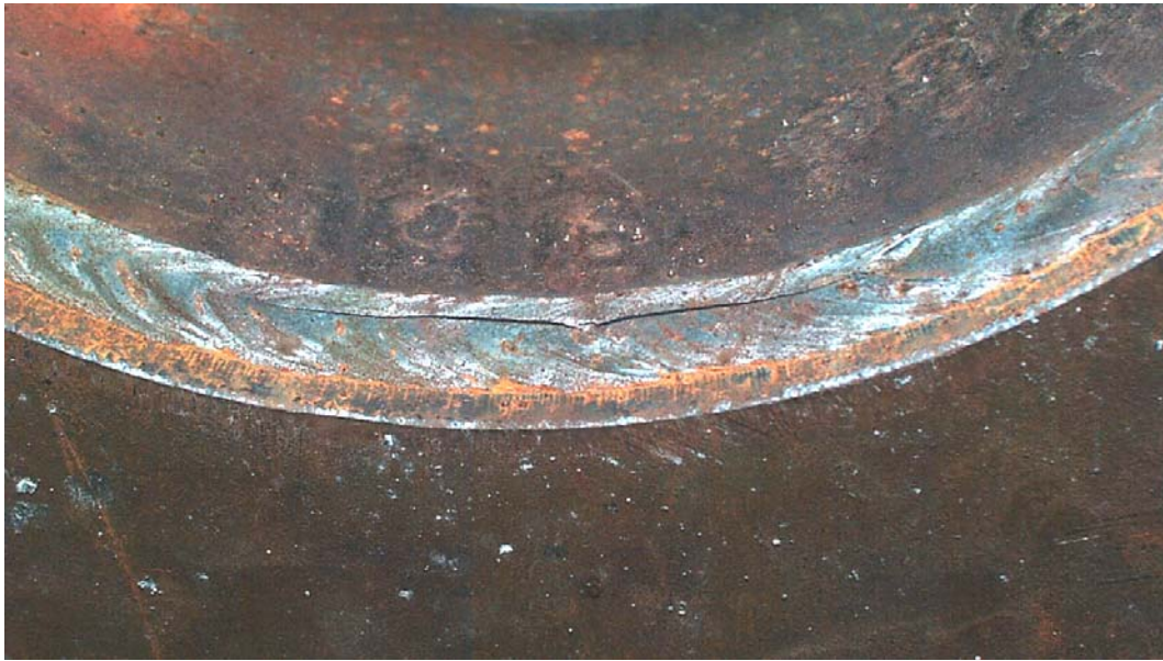
Figure 7.28 Crack Observed in Interior Weld of External Collar Stiffened Specimen
