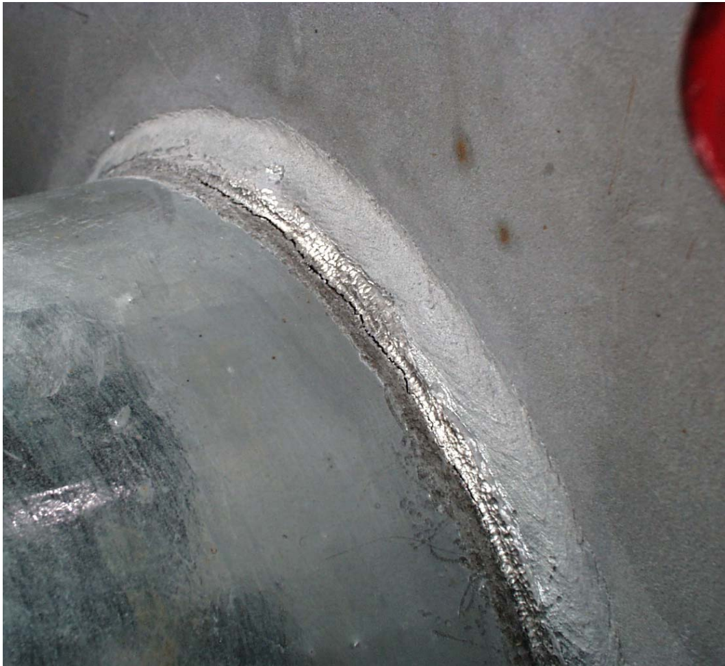
Figure 7.19 Failure of UIT Retrofit Specimen After Unloading and Retesting – VALNu PR ul Specimen
