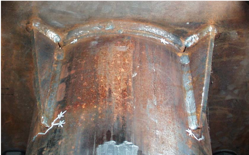
Figure 7.12 Failure of VALN 6x3/8@45 Specimen – Paint lines at termination of stiffeners represent extents of visible cracking, and painted arrows indicate visible crack tips in socket weld toe. Specimen tested at 12 ksi stress range.
