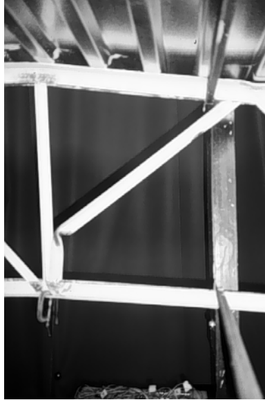
Figure 3.14 Failure Mode for 26K5-PW-1 East Joist
