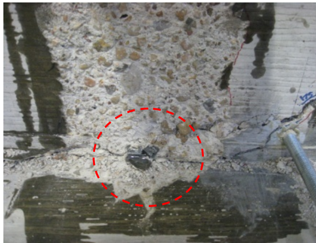
Figure 4-101 Anchor fracture in test 24-3-10
