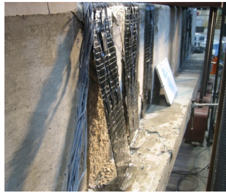
(b) Intermediate crack debonding
