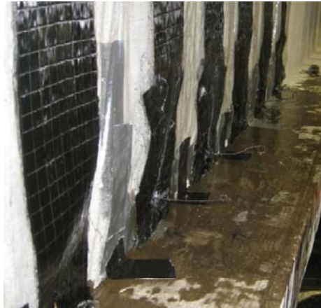
Figure 4-14 Poor application of CFRP strip and anchor due to plastic wrapping
