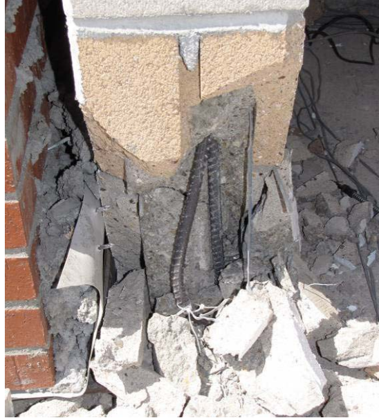
Figure 7-21 Inelastic buckling of splice in longitudinal reinforcement at west side of door on south side (2nd Tarzana 150 %)
