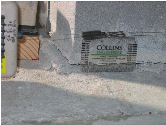
Figure 5-23 South end of CMU wall at the base under the first 1.0 in. loading to the north (Specimen UT CMU 4 MC)
