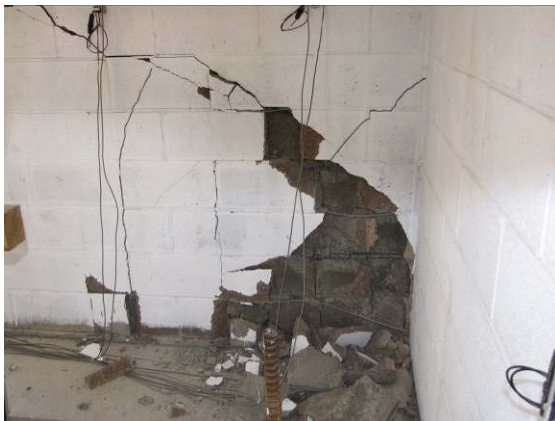
Figure 7-19 Damage to CMU at southeast corner (2nd Tarzana 150 %)
