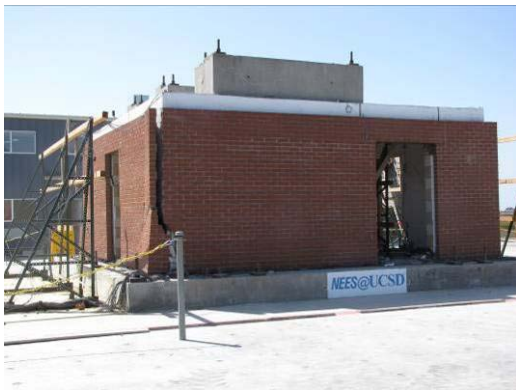
Figure 7-18 Damage to veneer on northeast corner and east side (2nd Tarzana 150 %)
