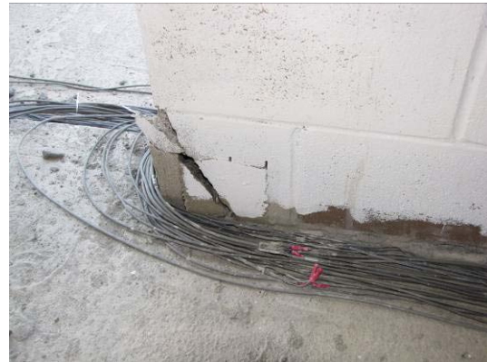
Figure 7-15 Local failure of CMU at edge of long segment on south side, due to in-plane sliding (1st Tarzana 150 %)
