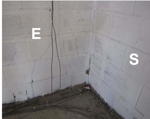
Figure 7-17 Flexural cracking of CMU wall at southeast corner due to out-of-plane flexure of horizontal wall strips as structure slid east-west (1st Tarzana 150 %)
