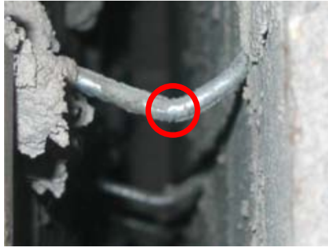
Figure 4-18 Cracked connector, second from the top, first from the west
