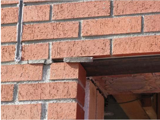
Figure 7-16 Relative displacement at expansion joint in clay veneer at door on South side (1st Tarzana 150 %)
