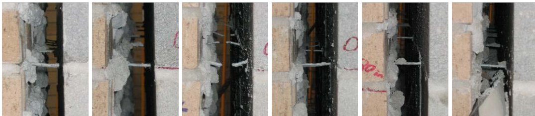
Figure 4-26 Connectors of UT CMU 2 MC at 0.8-in. tensile displacement (top to bottom, west side)
