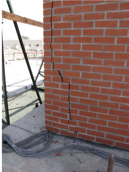
Figure 7-13 Cracking of veneer at northeast corner (1st Tarzana 150 %)
