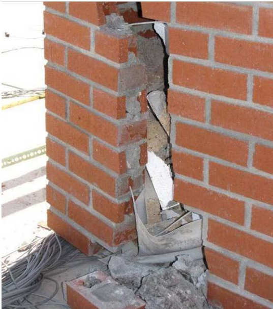
Figure 7-22 Detail of damage to northeast corner (2nd Tarzana 150 %)
