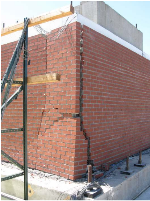
Figure 7-30 Northeast corner (2nd Tarzana 150 %)
