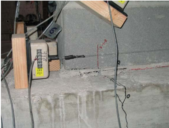
Figure 5-17 South end of CMU wall at the base under the first 1.0 in. loading to the north (Specimen UT CMU 4)
