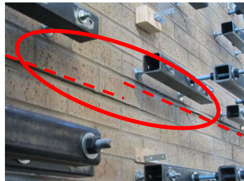
Figure 4-20 Joining of cracks in the clay masonry veneer
