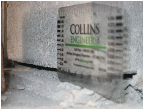
Figure 5-11 South end of CMU wall at the base under the first 1.0 in. loading to the north (Specimen UT CMU 3)
