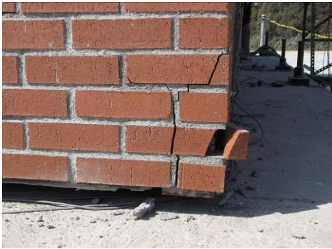
Figure 7-14 Cracking of veneer at southeast corner (1st Tarzana 150 %)
