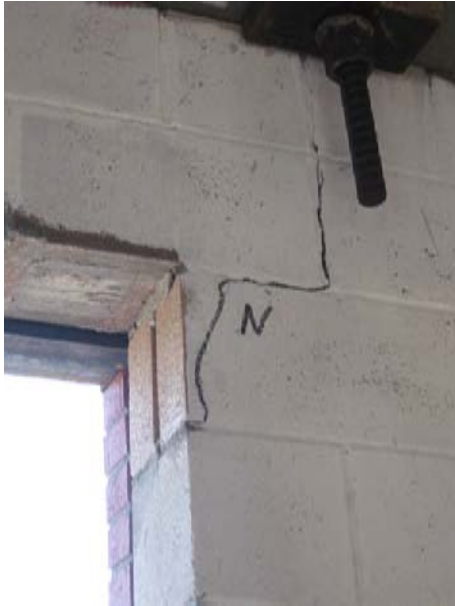
Figure 7-12 Cracking near lintel end on north side (1st Tarzana 150 %)
