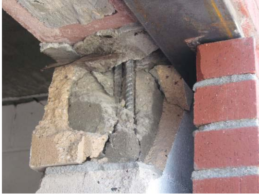
Figure 7-20 Damage to lintel over door on north side (2nd Tarzana 150 %)
