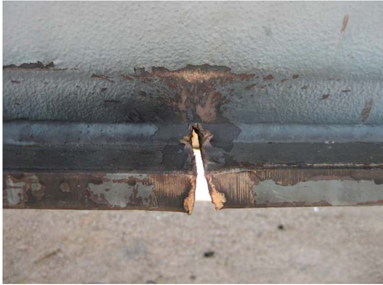
Figure 3-14: Bottom flange, post-fracture
