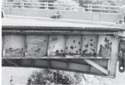
Figure 2-4: Mianus River Bridge, post-collapse (Fisher 2005)
