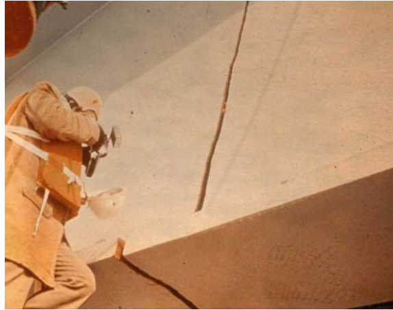
Figure 2-5: Full-depth fracture in I-79 bridge in Pittsburg, PA (unknown)
