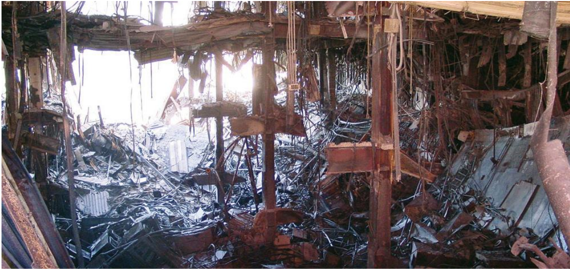
Figure 1.2 Connection failure at tree column of WTC5 (FEMA 2002)
