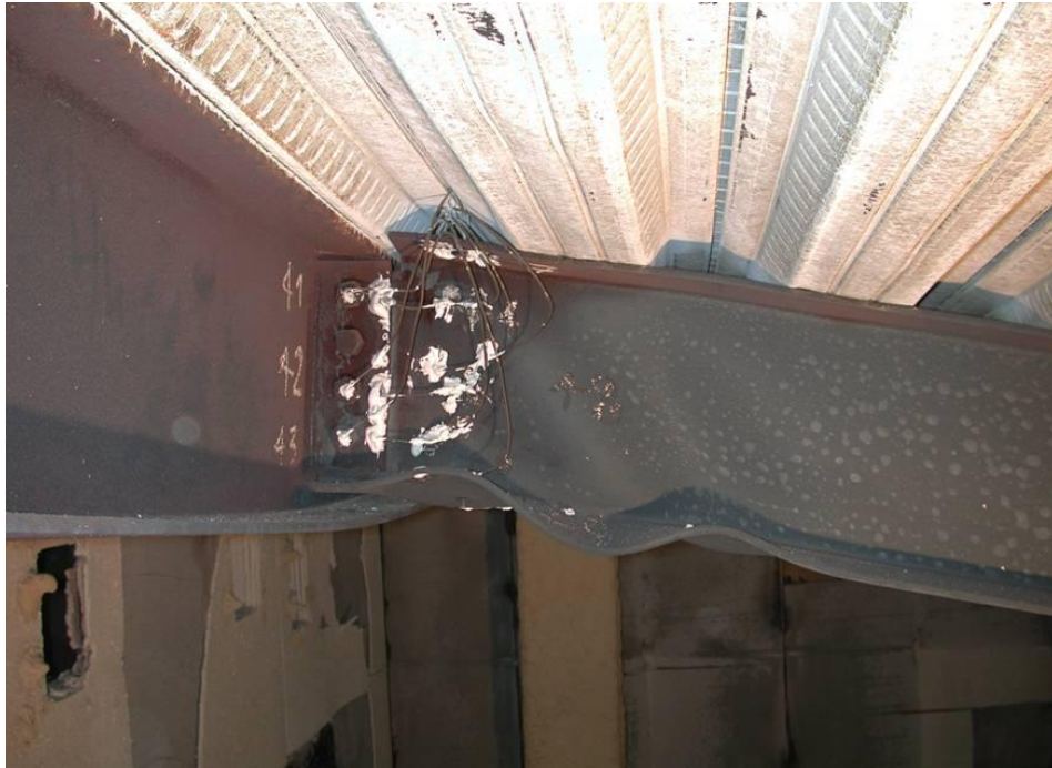
Figure 1.5 Simple shear beam end connection damage in fire (Cardington test report 2003)
