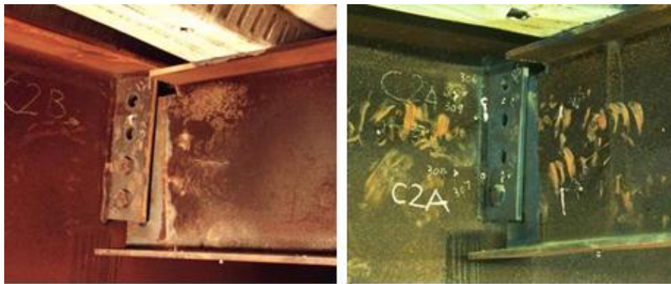
Figure 1.4 Simple shear beam end framing connection damage in heating (left) and cooling (right) (Cardington test report 1998)
