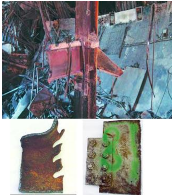
Figure 1.3 Connection tear out failure in WTC5 (FEMA 2002)
