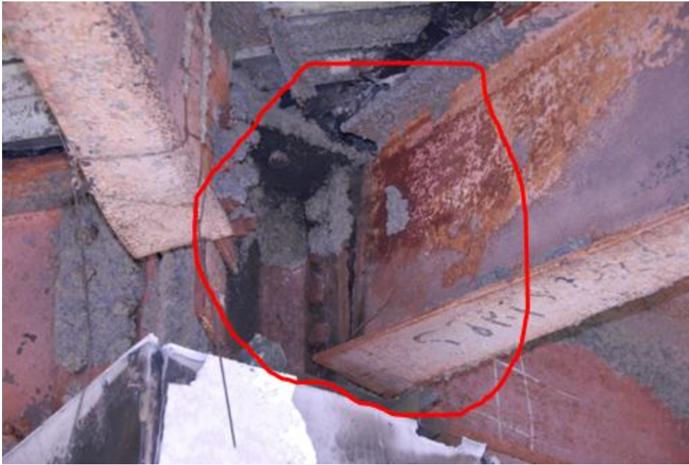
Figure 1.8 Connection damage in Echelon Building due to fire
