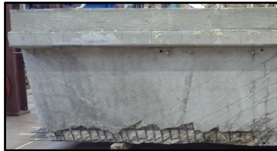
(B) Horizontal shear failure in Texas U54
