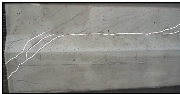
(C) Horizontal shear distress in Texas 5B40 (Avendaño, 2011)
