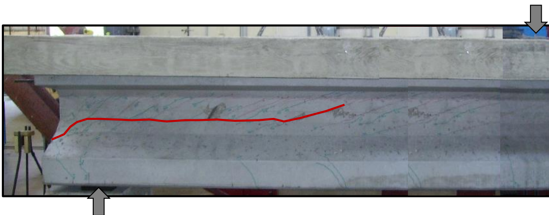
Figure 2-16: Tx28 after shear testing, with horizontal failure crack highlighted.
